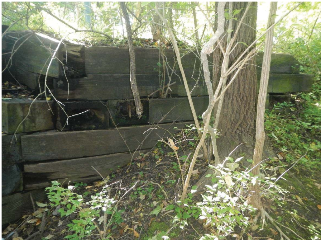
30. Near (West) Abutment Left (North) Wing Decay
