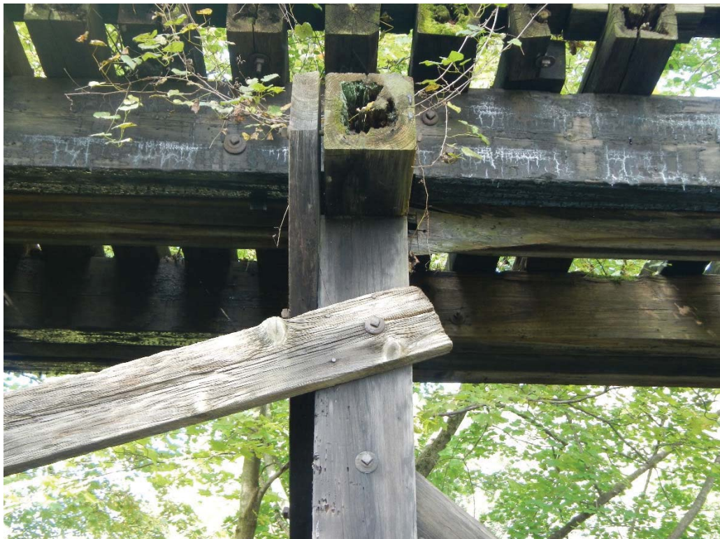
44. Pier 3 Right (South) End Top Strut Decay
