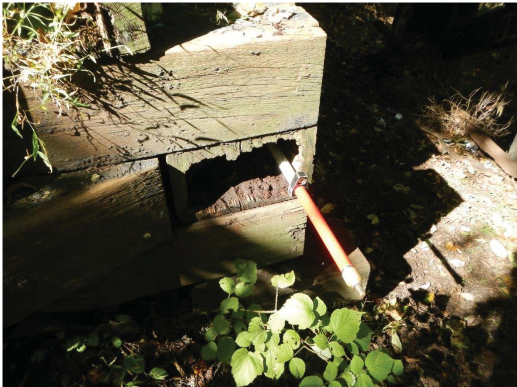
26. Near (West) Abutment Stem Transverse Member Decay (3' of Penetration with 4' Rod)
