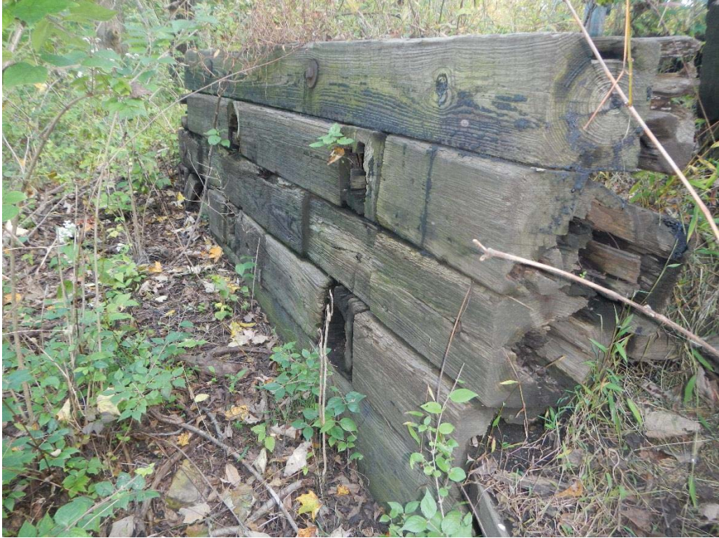
31. Far (East) Abutment Left (North) Wing Decay
