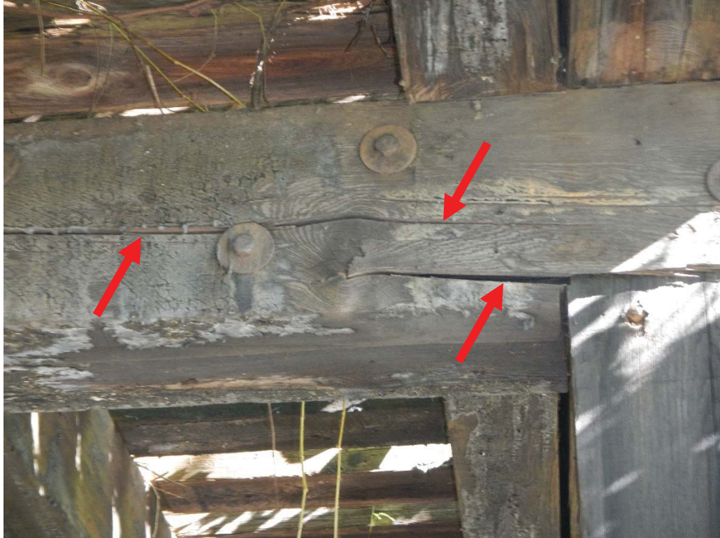
45. Pier 13 Near (West) Face Top Strut Splits
