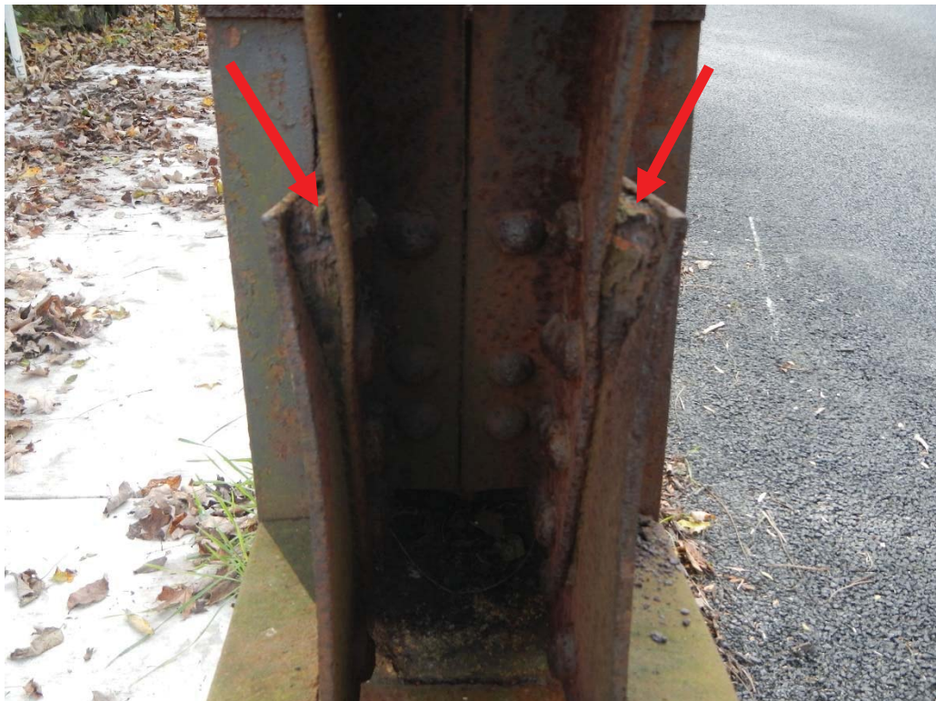
70. Pier 7 Column 1 Bracing Vertical Gusset Plates Bent with Pack Rust
