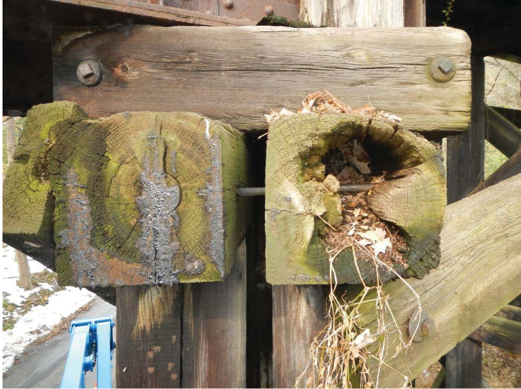
39. Pier 5 Right (South) End Top Strut Decay
