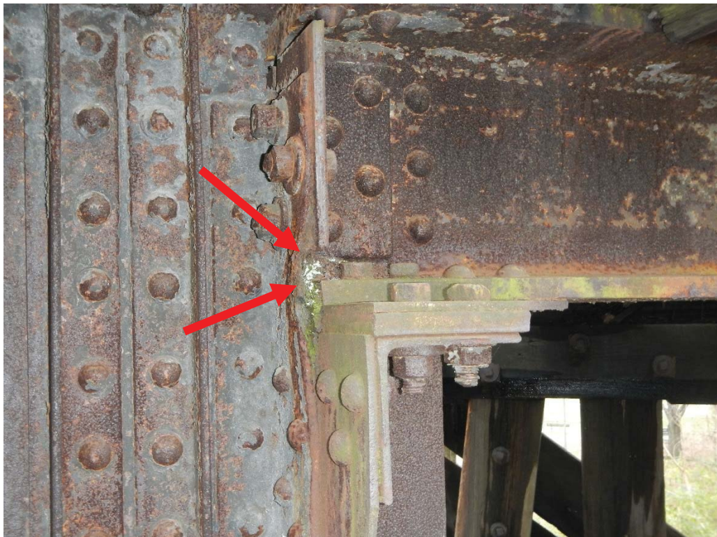
28. Span 7 Stringer 1 100% Section Loss to Connection Angle Adjacent to Pier 7
