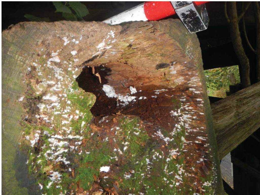
36. Pier 2 Right (South) End Top Strut Decay and Algae/Fungus Growth Close Up
