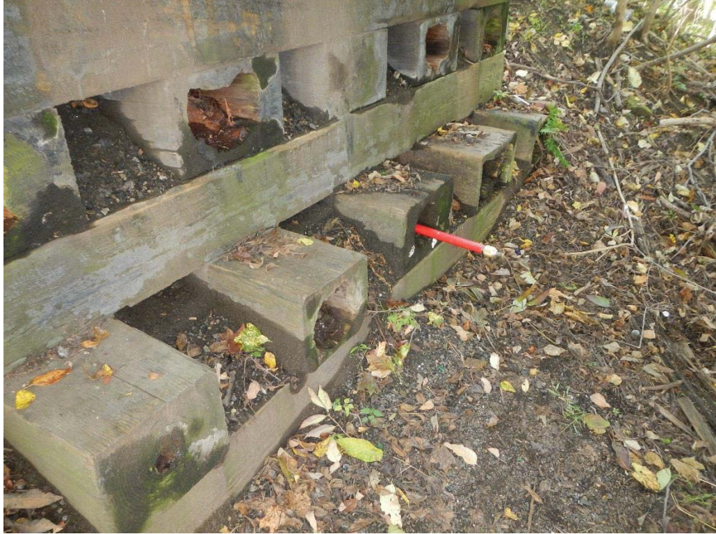
25. Near (West) Abutment Stem Longitudinal Member Decay (3' of Penetration with 4' Rod, Typical Condition)
