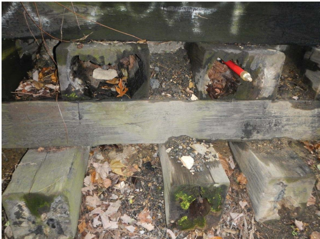
28. Far (East) Abutment Stem Longitudinal Member Decay (3'-6" of Penetration with 4' Rod, Typical Condition)
