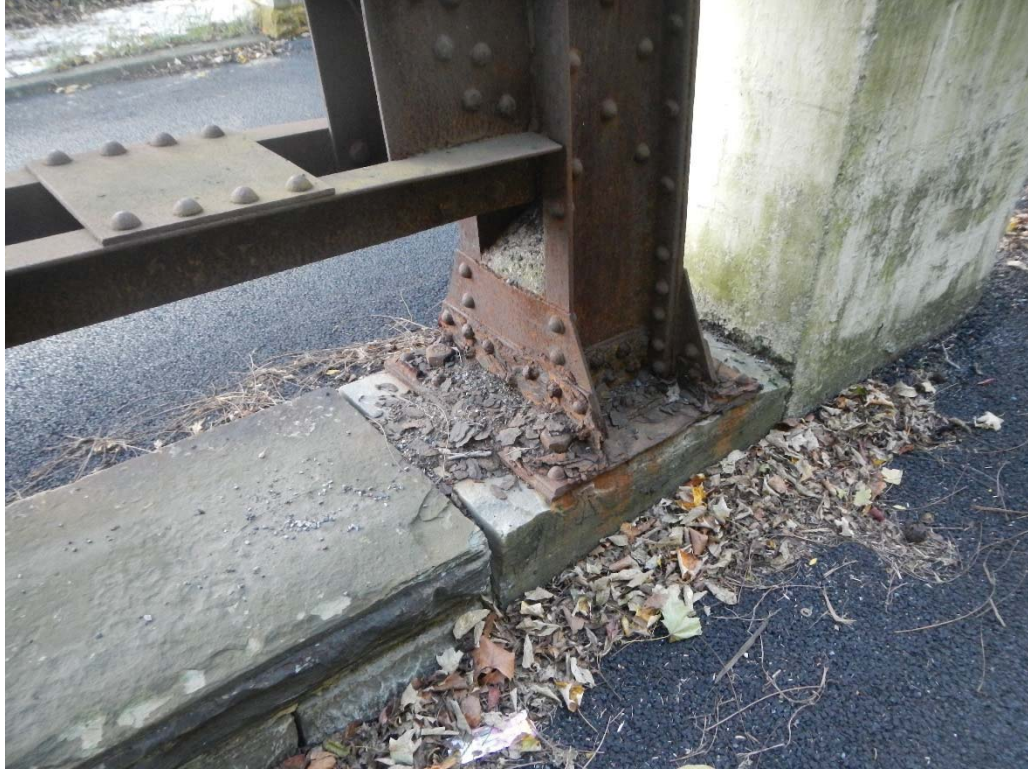
73. Pier 8 Column 1 Connection Angle Section Loss
