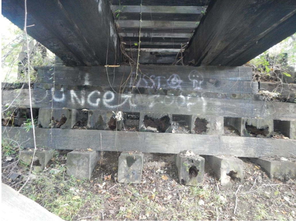
27. General View of Far (East) Abutment Stem Longitudinal Member Decay
