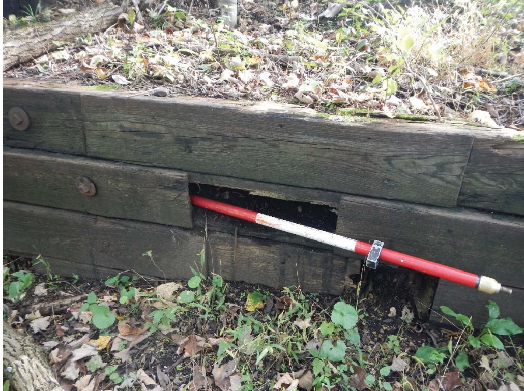
39. Near (West) Abutment Left (North) Wing Decay
