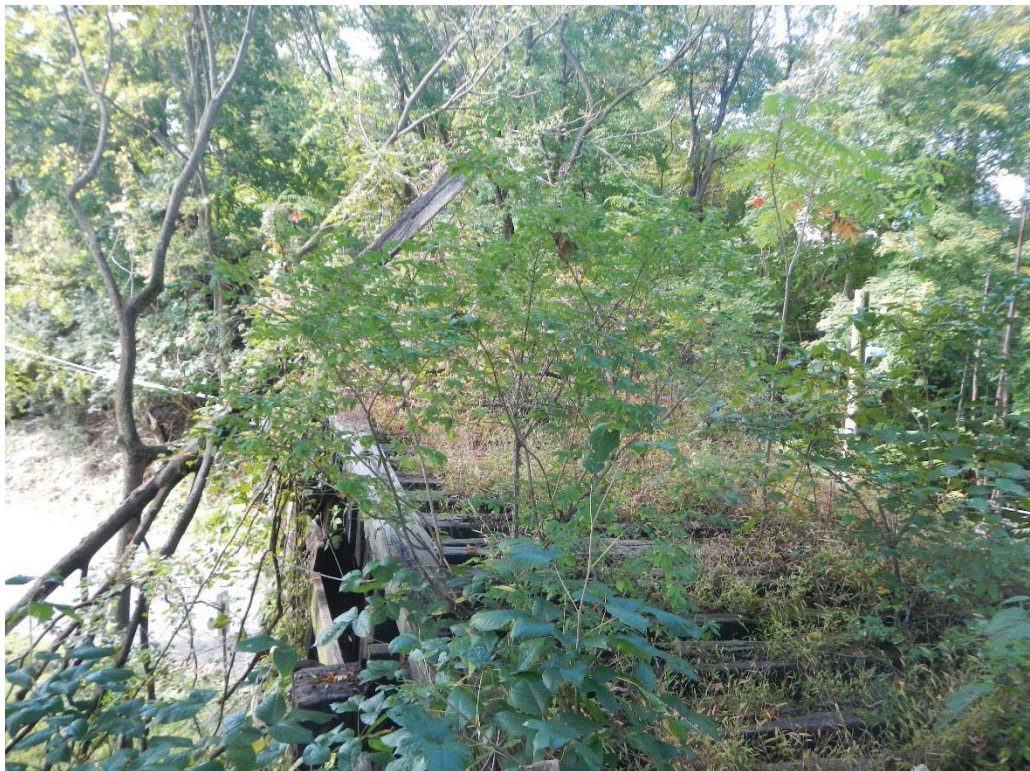
12. Significant Vegetation Growth Along Ties at Far (East) End
