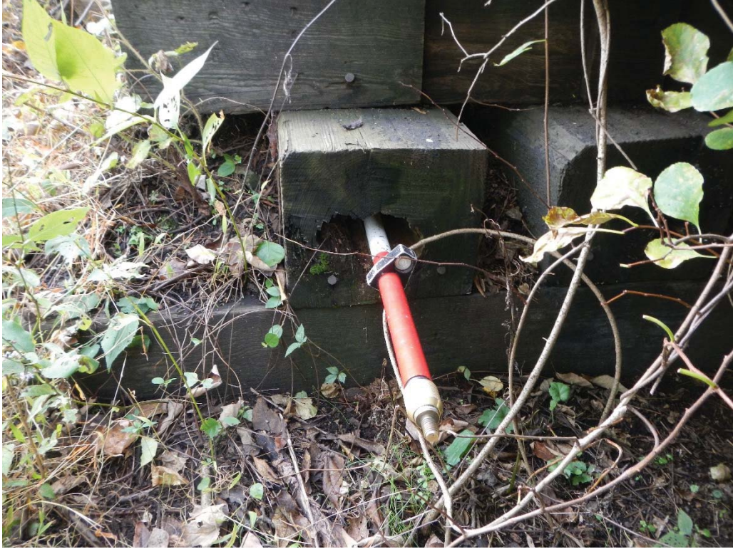
37. Near (West) Abutment Stem Longitudinal Member Decay (3' of Penetration with 4' Rod)
