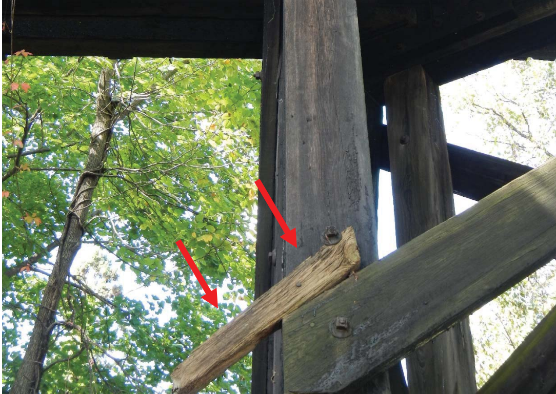
65. Span 5 Right (South) Longitudinal Bracing Missing at Pier 5
