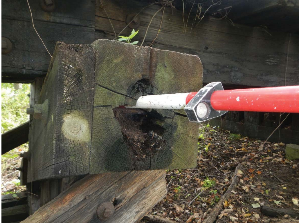
43. Pier 1 Left (North) End Top Strut Decay (2'-4" Penetration with 4' Rod)
