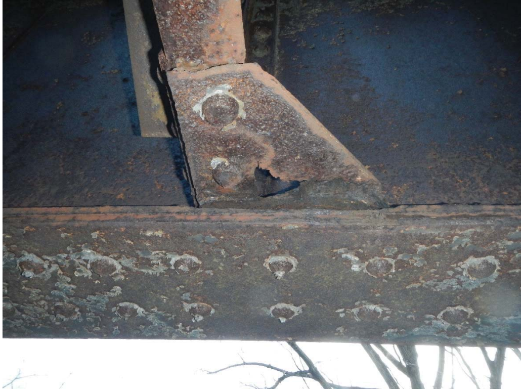
31. Span 8 Girder 2 Bottom Flange 100% Section Loss to Horizontal Gusset Plate at Diaphragm 3
