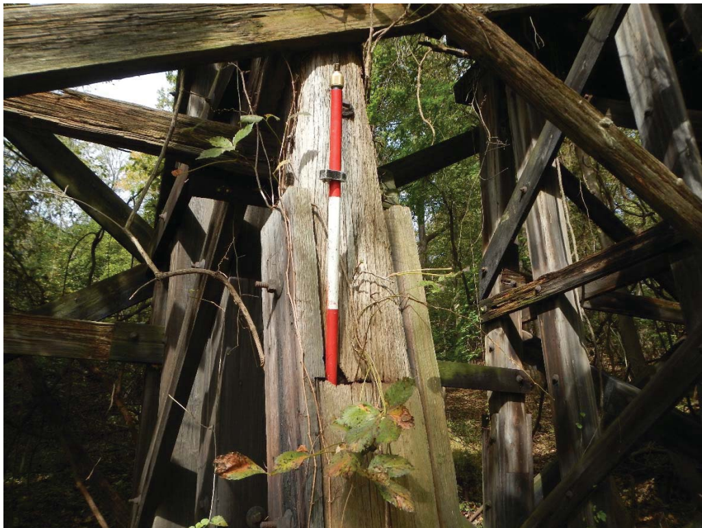
54. Pier 14 Column 4 Decay Around Column Splice (1'-4" of Penetration with 4' Rod)
