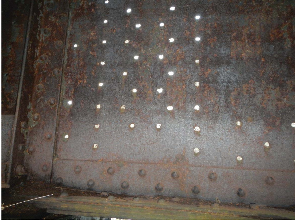
23. Open Bolt Holes in Girder 1 Web Near Pier 4
