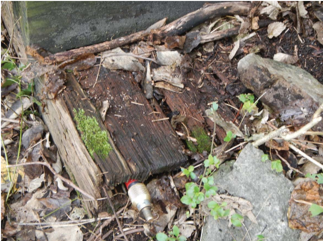
64. Pier 17 Right (South) End Footing Decay (4' of Penetration with 4' Rod)
