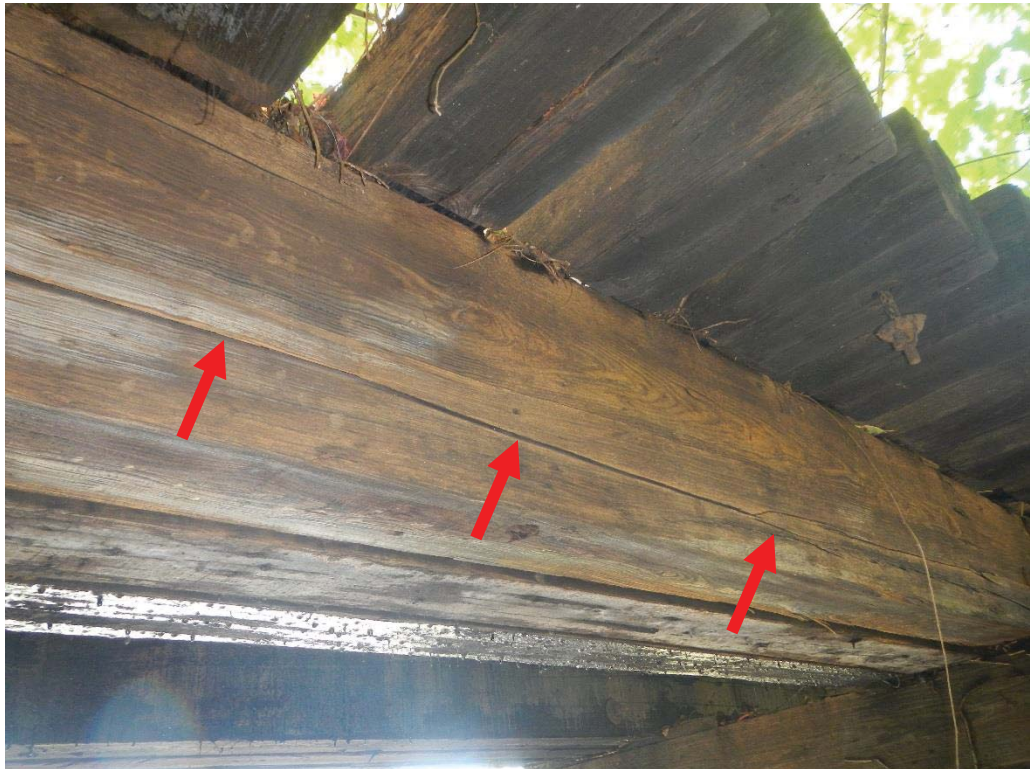
20. Span 13 Stringer 1 Horizontal Split in Stringer
