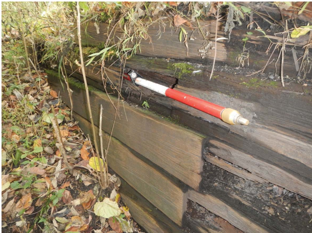
40. Far (East) Abutment Left (North) Wing Decay
