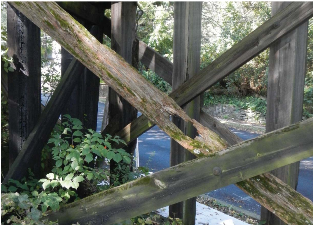
66. Span 6 Right (South) Longitudinal Bracing Decay
