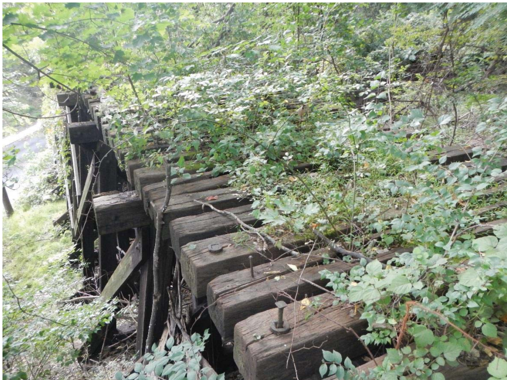
14. Significant Vegetation Growth Along Ties at Far (East) End
