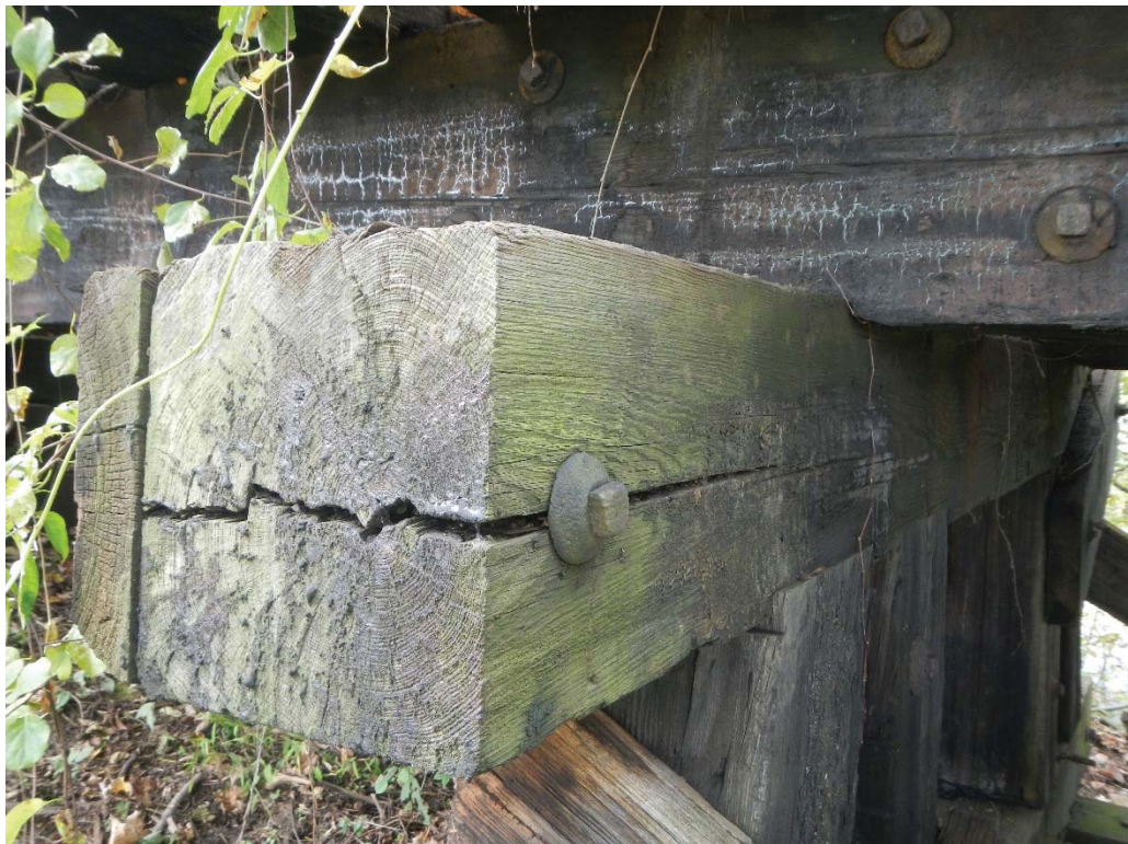
42. Pier 1 Right (South) End Top Strut Split (Split is Full Length)
