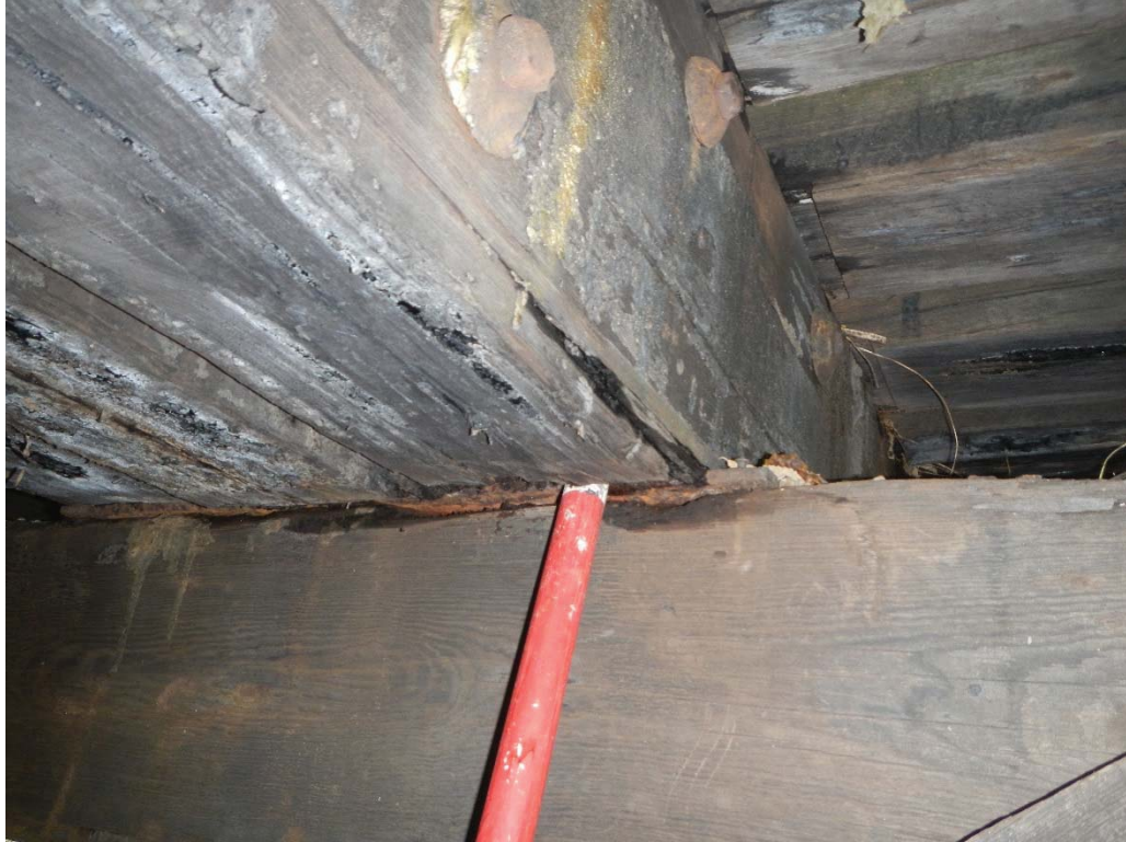
27. Span 19 Stringer 1 Decay to Bottom of Stringer Adj to Pier 18 (1' of Penetration with Rod) (Decay Extends Full Height)
