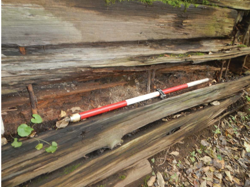
41. Far (East) Abutment Right (South) Wing Decay
