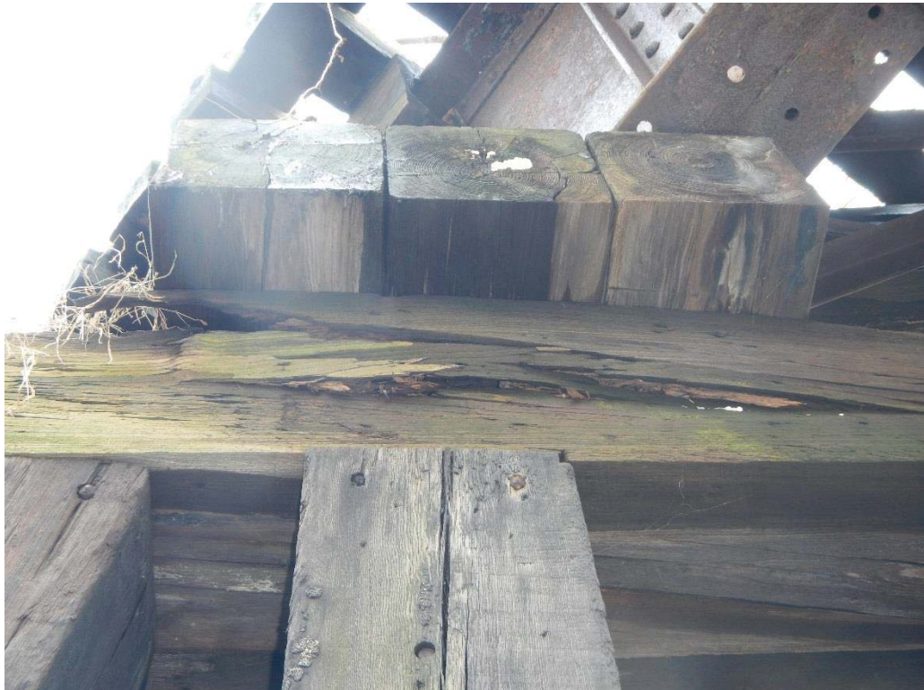
38. Pier 5 Near (West) Side Top Strut Decay Over Column 2 (Decay Extends to Left (North) End)
