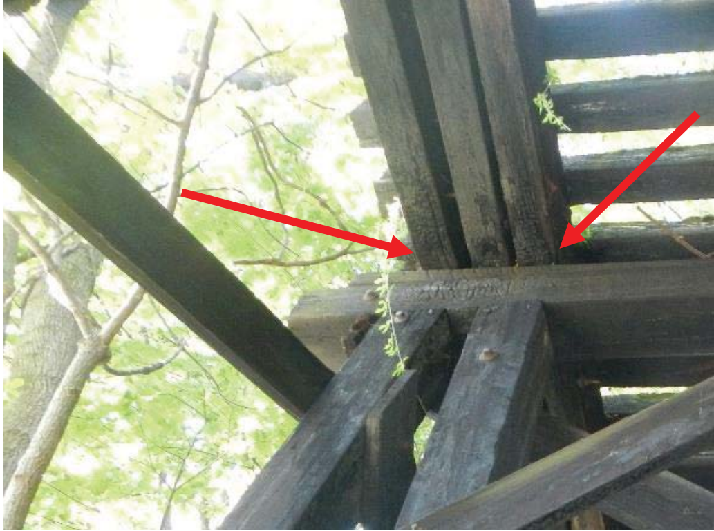
17. Span 4 Stringers 4 Thru 6 Fire/Fungus Damage Along Bottom of Stringers Adjacent to Pier 3
