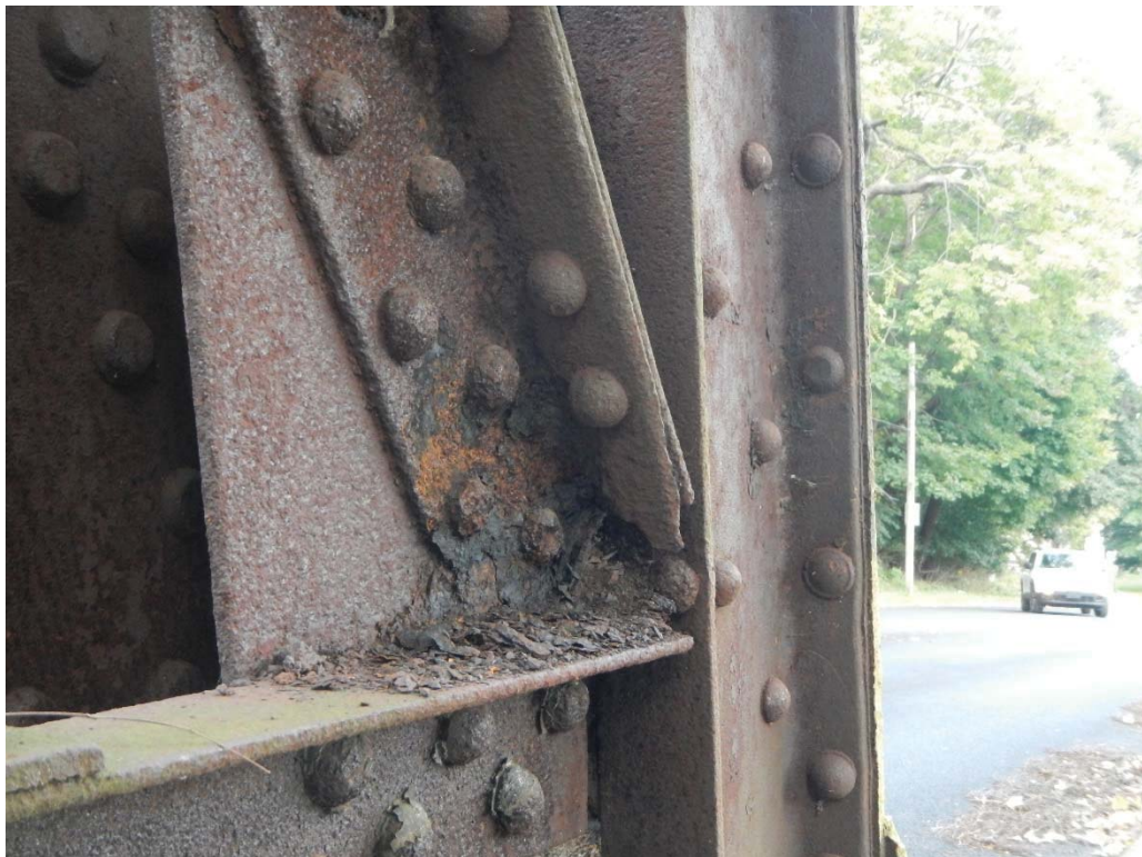
72. Pier 7 Column 2 Near (West) Bracing 100% Section Loss
