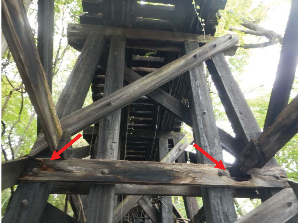
69. Pier 16 Near (West) Horizontal Transverse Brace Decay
