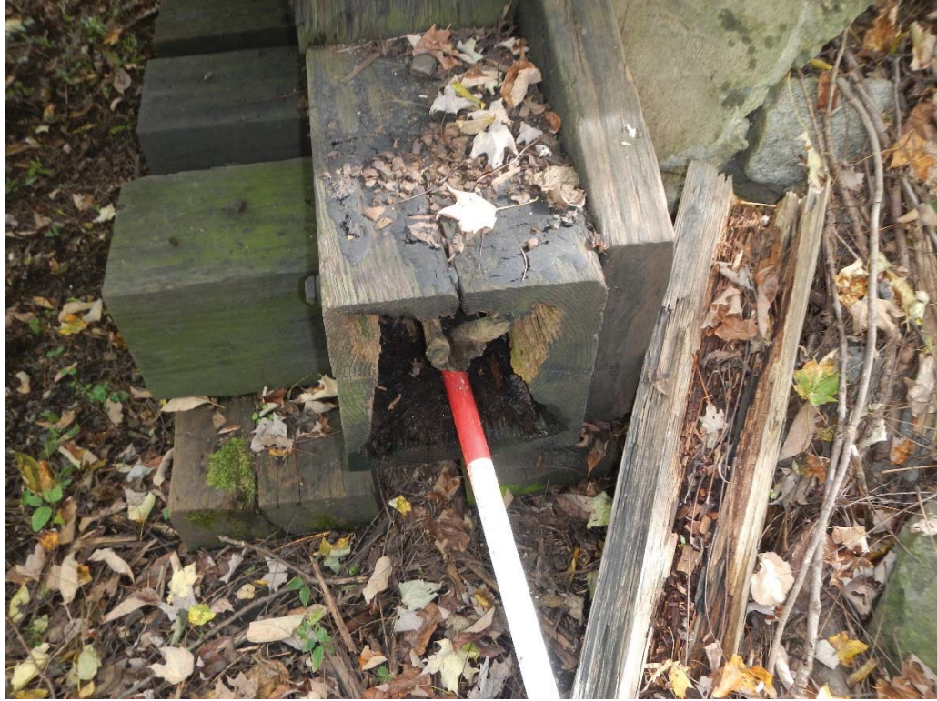
57. Pier 1 Left (North) End Bottom Strut Decay (2' of Penetration with 4' Rod)
