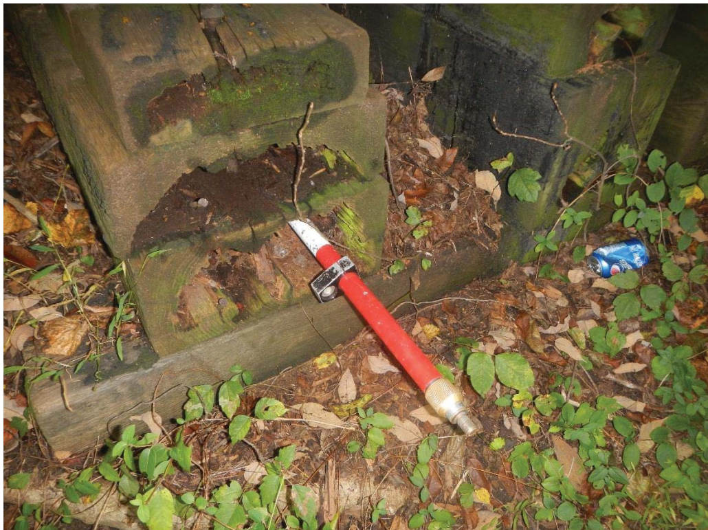
50. Pier 2 Mudsill 8 Decay Close Up (3' of Penetration with 4' Rod, Typical Condition)
