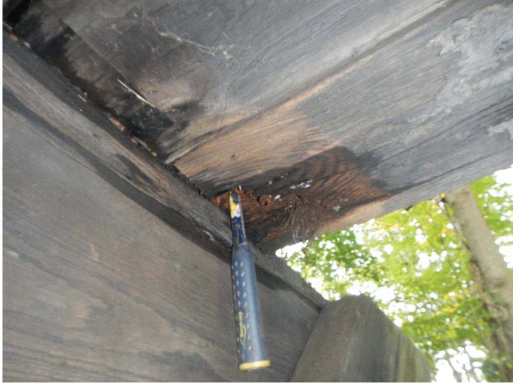
15. Span 3 Stringer 1 Decay at Bot of Stringer Adj to Pier 2 (Hammer Penetration up to 6") (Decay Extends Full Height)
