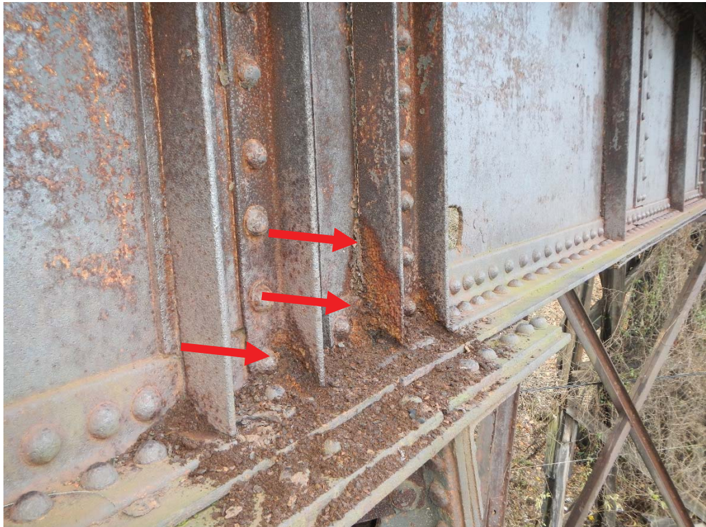
32. Span 8 Girder 2 Section Loss to Exterior Stiffeners Adjacent to Pier 8
