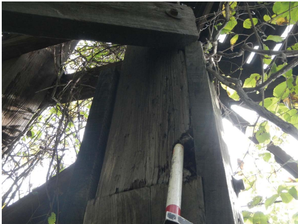
50. Pier 10 Column 1 Decay Around Column Splice
