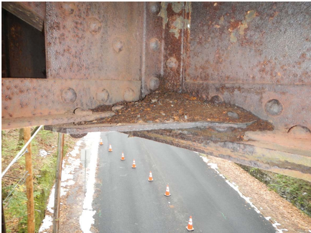
30. Span 8 Girder 1 Bottom Flange Steel Rust Residue on Horizontal Gusset Plate (Typical)
