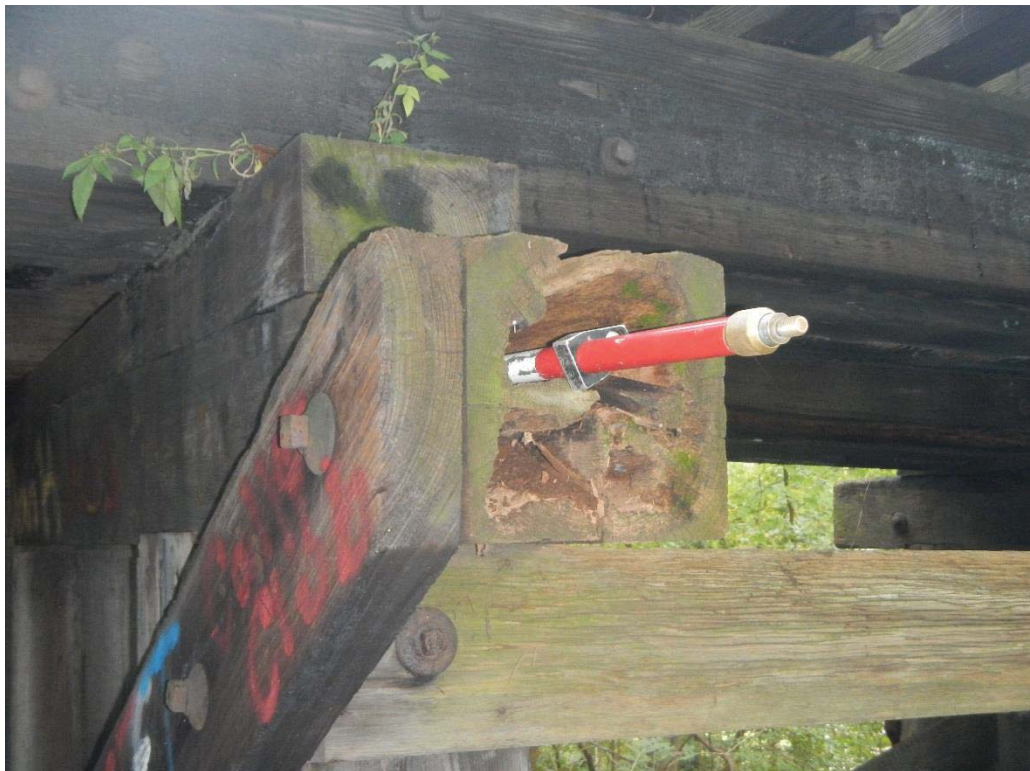
34. Pier 1 Right (South) End Top Strut Decay Close Up (3'-2" of Penetration with 4' Rod)
