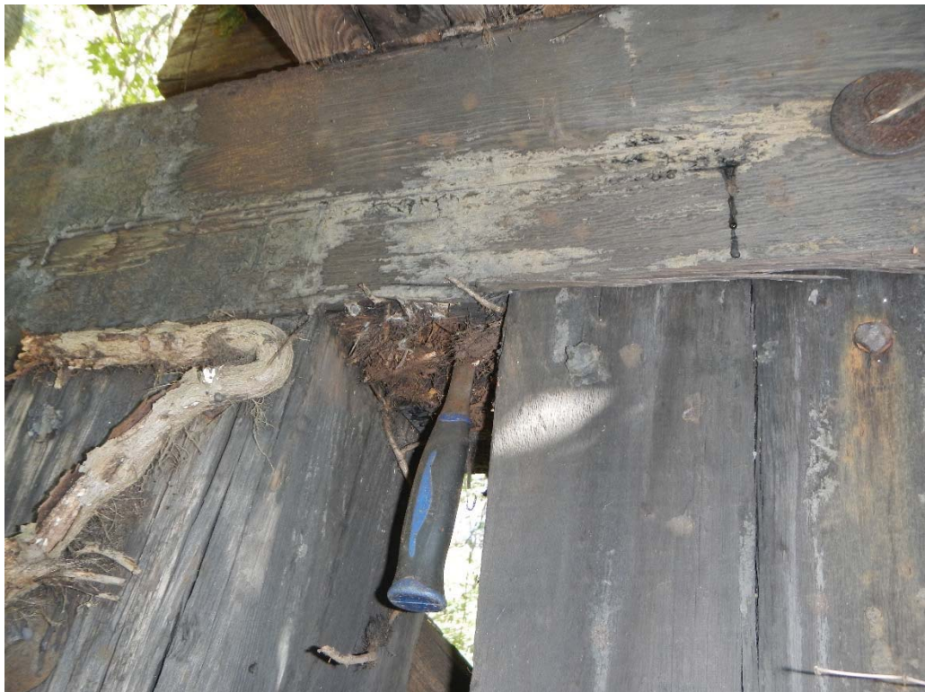
46. Pier 13 Near (West) Side Top Strut Decay Btw Cols 1 and 2 (Hammer Penetration up to 6") (Decay Extends Full Height)
