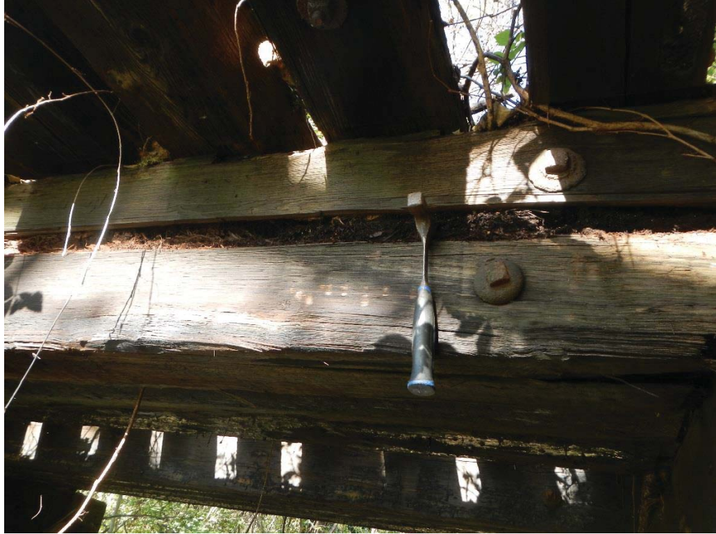
23. Span 15 Stringer 6 Decay to Stringer Along Entire Span Close Up
