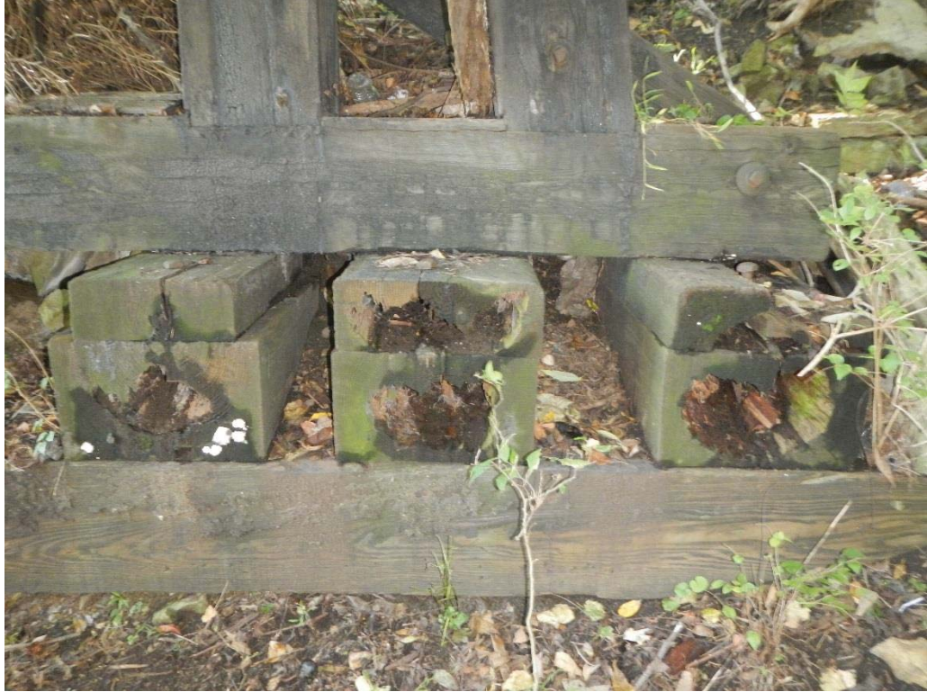
47. Pier 1 Mudsills 1 thru 3 Decay (Typical Condition)
