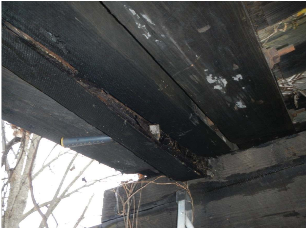
20. Span 8 Stringer 5 Decay to Bottom of Stringer Adjacent to Pier 7
