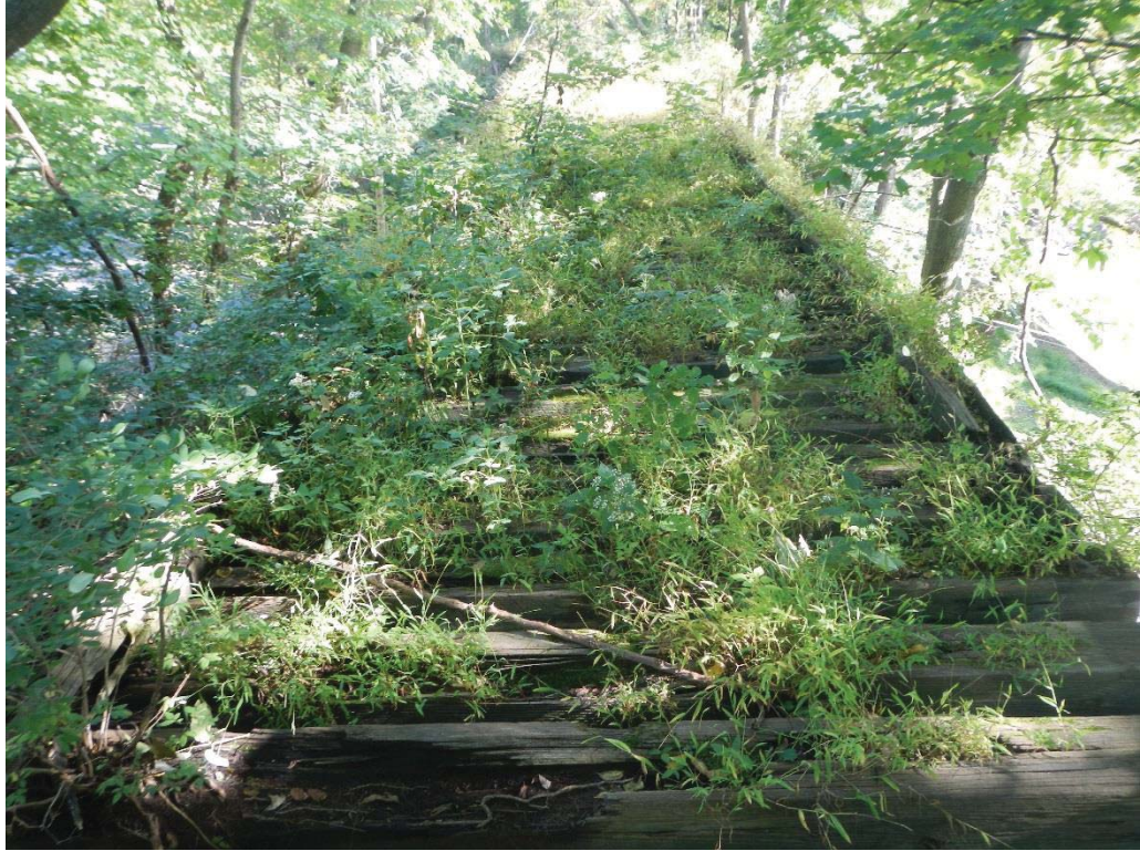
11. Significant Vegetation Growth Along Ties at Near (West) End
