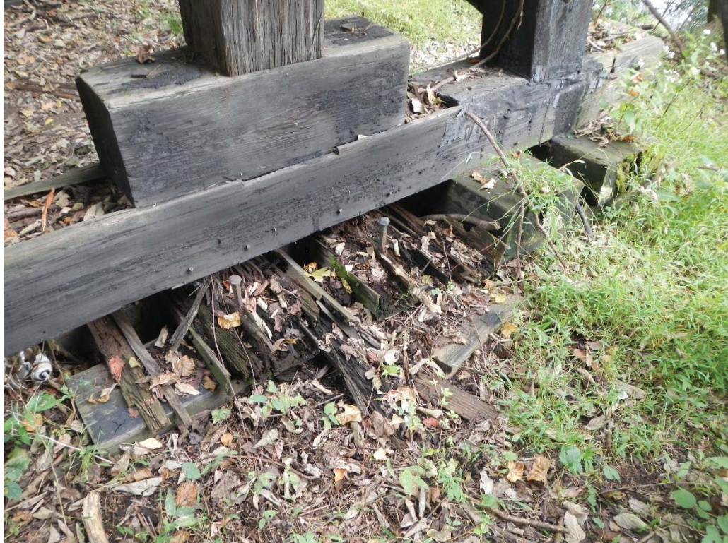
61. Pier 15 Mudsills 5 thru 8 Decay (Typical Condition)
