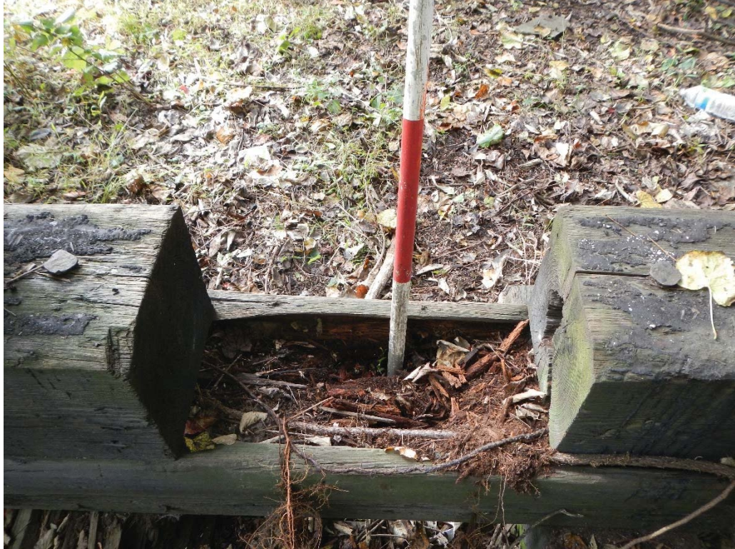
59. Pier 15 Bottom Strut Decay Between Columns 2 and 3 (Decay Extends Full Length)
