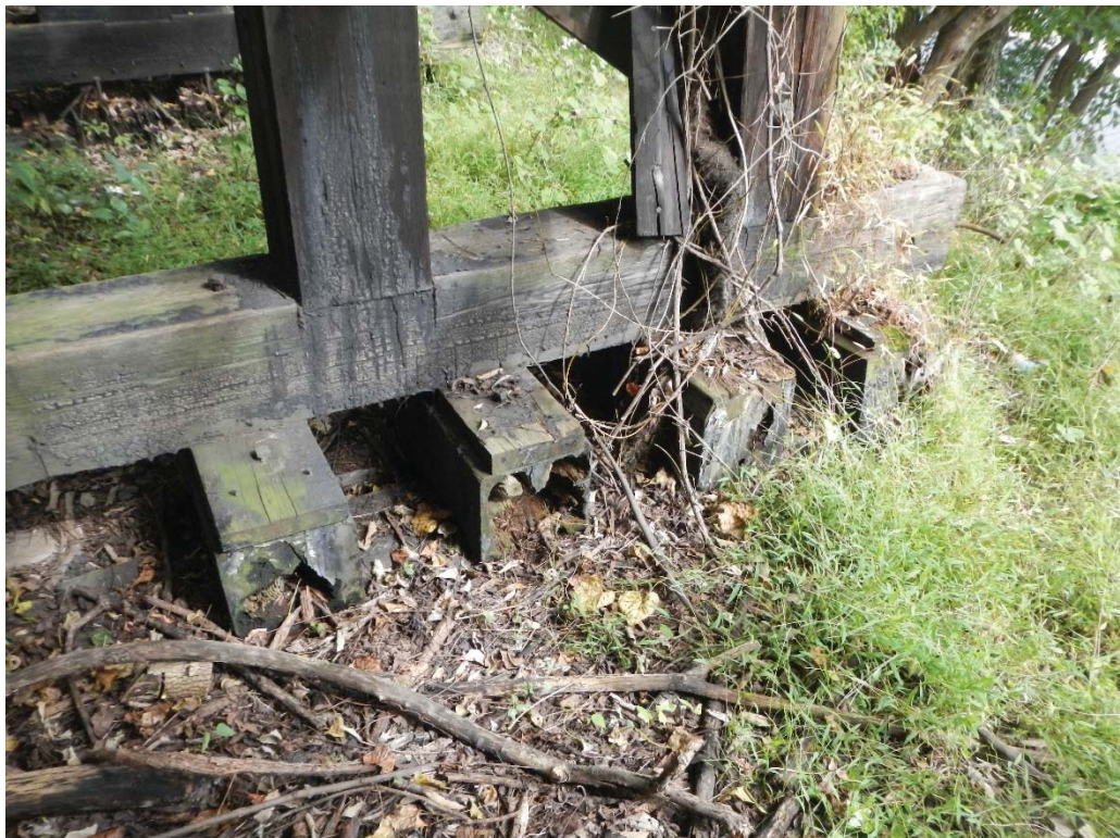
60. Pier 14 Mudsills 5 thru 8 Decay (Typical Condition)
