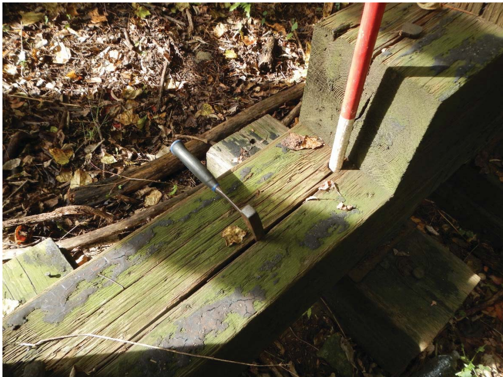
58. Pier 14 Bottom Strut Split/Decay
