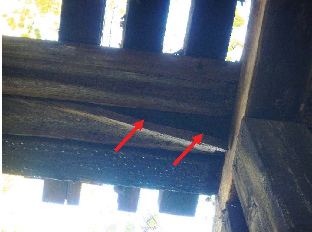
17. Span 4 Stringer 5 Decay Along Bottom of Stringer Adjacent to Pier 3 (Decay Extends Full Length)
