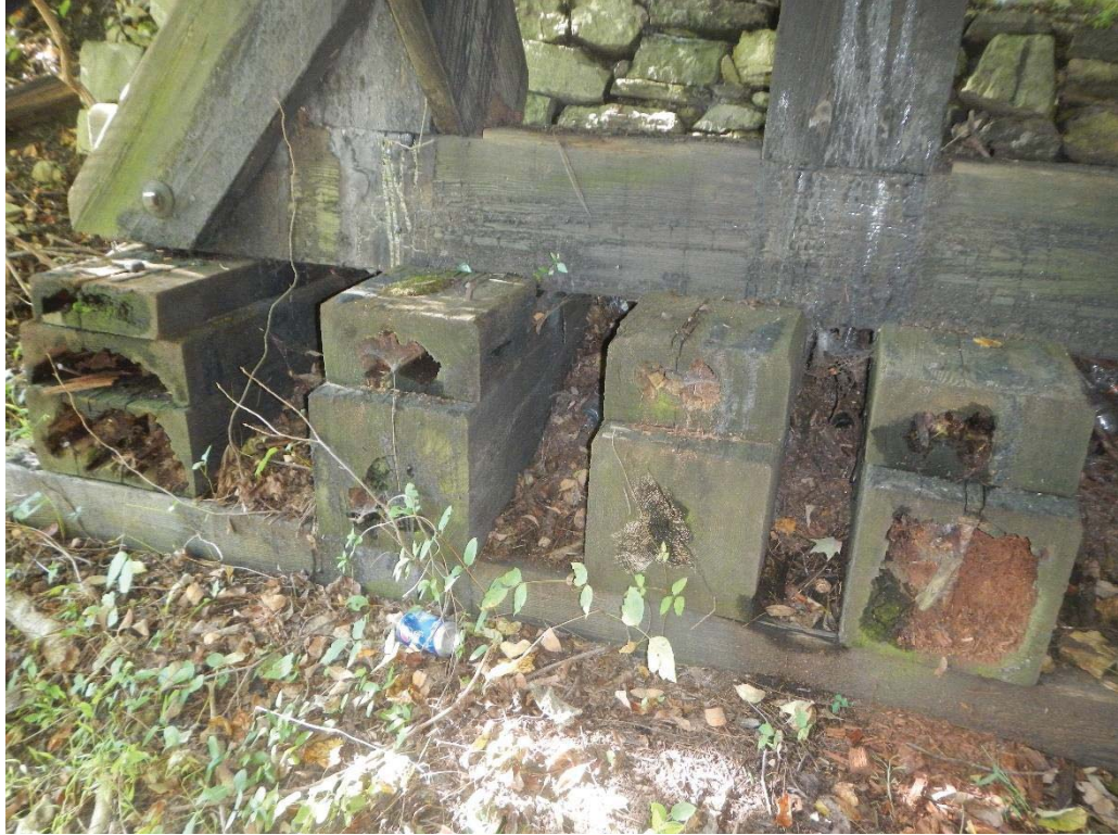
49. Pier 2 Mudsills 5 thru 8 Decay (Typical Condition)
