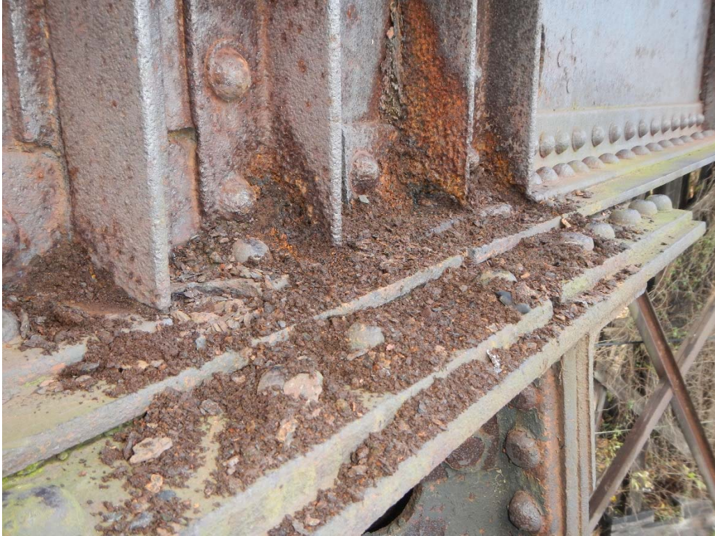
33. Span 8 Girder 2 Section Loss to Exterior Stiffeners Adjacent to Pier 8 Close Up
