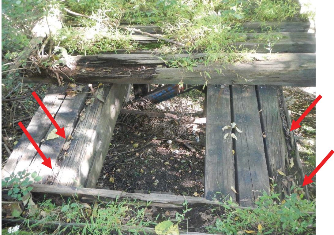
13. Span 1 Stringers Decay to Top of Stringers Adjacent to Near (West) Abutment
