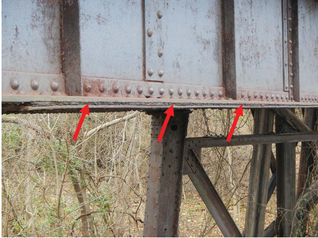
35. Span 9 Girder 2 Pack Rust Between Bottom Flange and Cover Plate (Typical)
