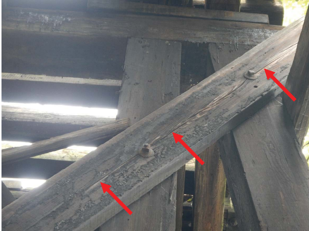
67. Pier 5 Near (West) Top Diagonal Transverse Brace Split
