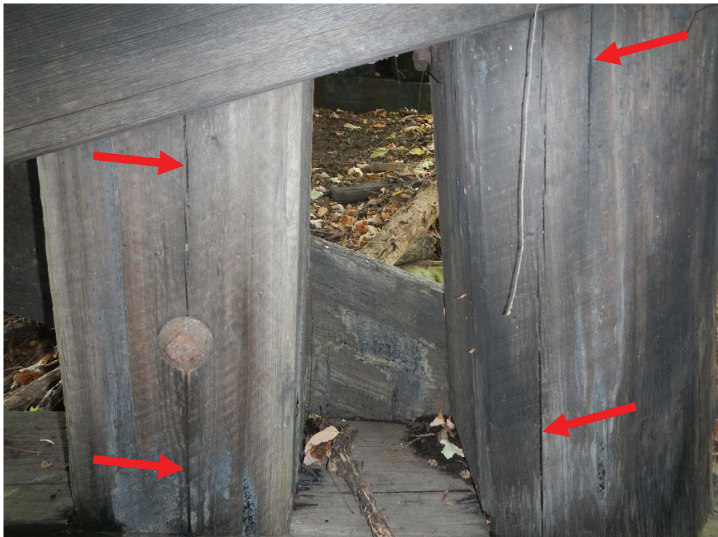
48. Pier 1 Columns 1 and 2 Splits Far (East) Face
