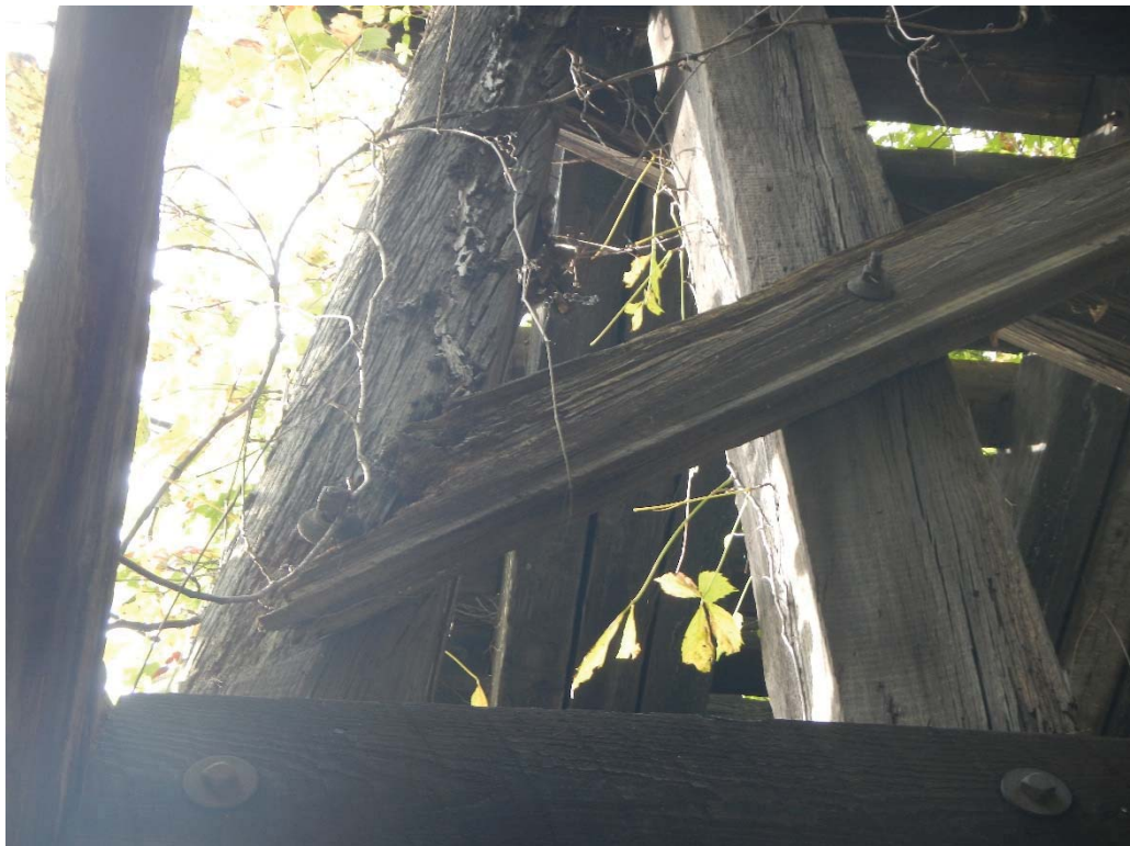
68. Pier 14 Far (East) Top Diagonal Transverse Brace Decay
