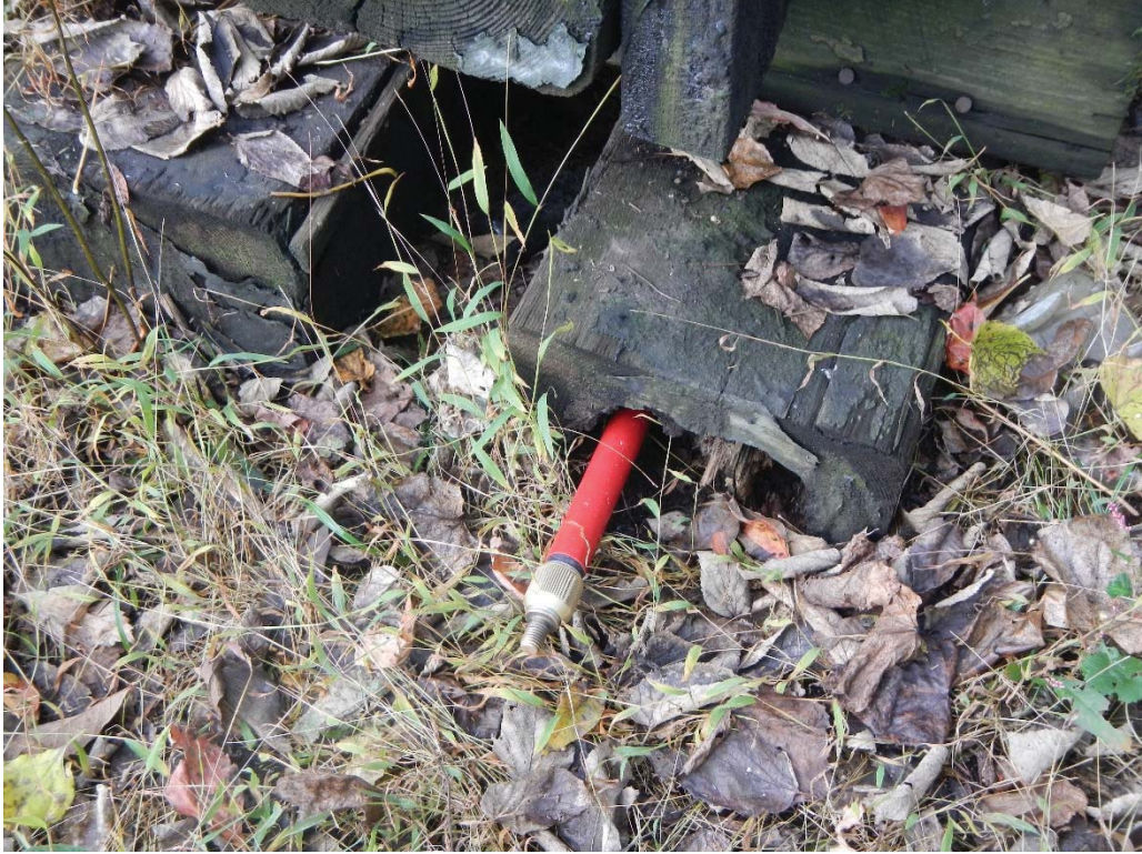
63. Pier 15 Far (East) Right (South) End Footing Decay (3'-6" Penetration with 4' Rod)
