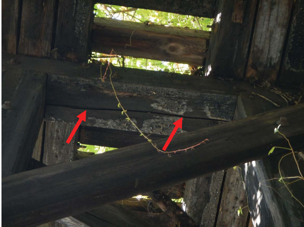
47. Pier 13 Top Strut Split at Underside Between Columns 2 and 3
