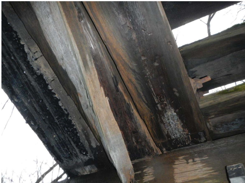
18. Span 4 Stringer 5 Decay Along Bottom of Stringer Adjacent to Pier 3 (Decay Extends Full Length) Close Up
