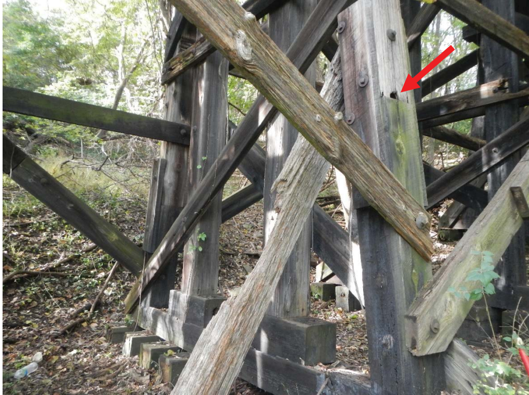
55. Pier 15 Column 4 Decay Around Column Splice
