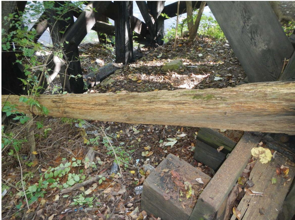
52. Span 3 Bottom Left (North) Longitudinal Bracing Weathering/Decay
