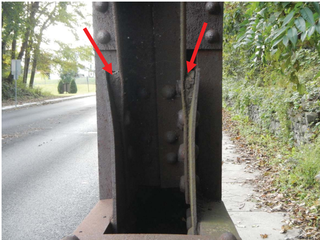
74. Pier 9 Column 1 Bracing Vertical Gusset Plates Bent with Pack Rust
