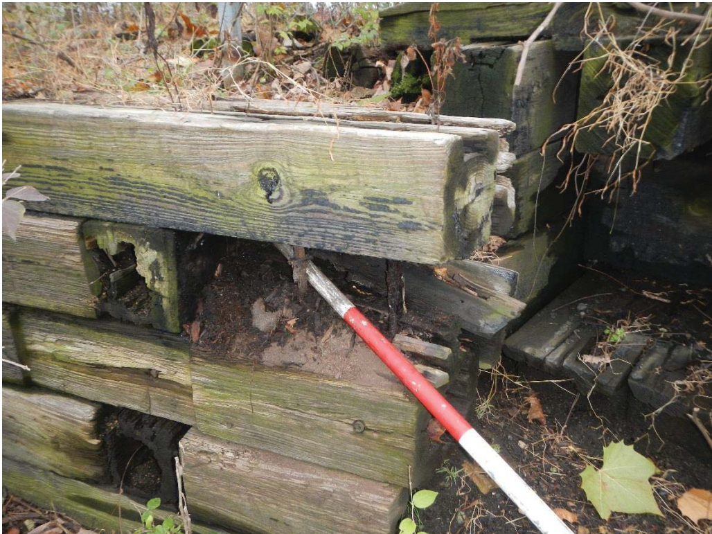
32. Far (East) Abutment Left (North) Wing Decay
