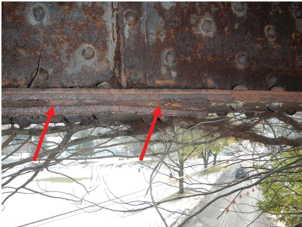
24. Pack Rust Between Girder 2 Cover Plates and Bent Cover Plate Near Pier 4
