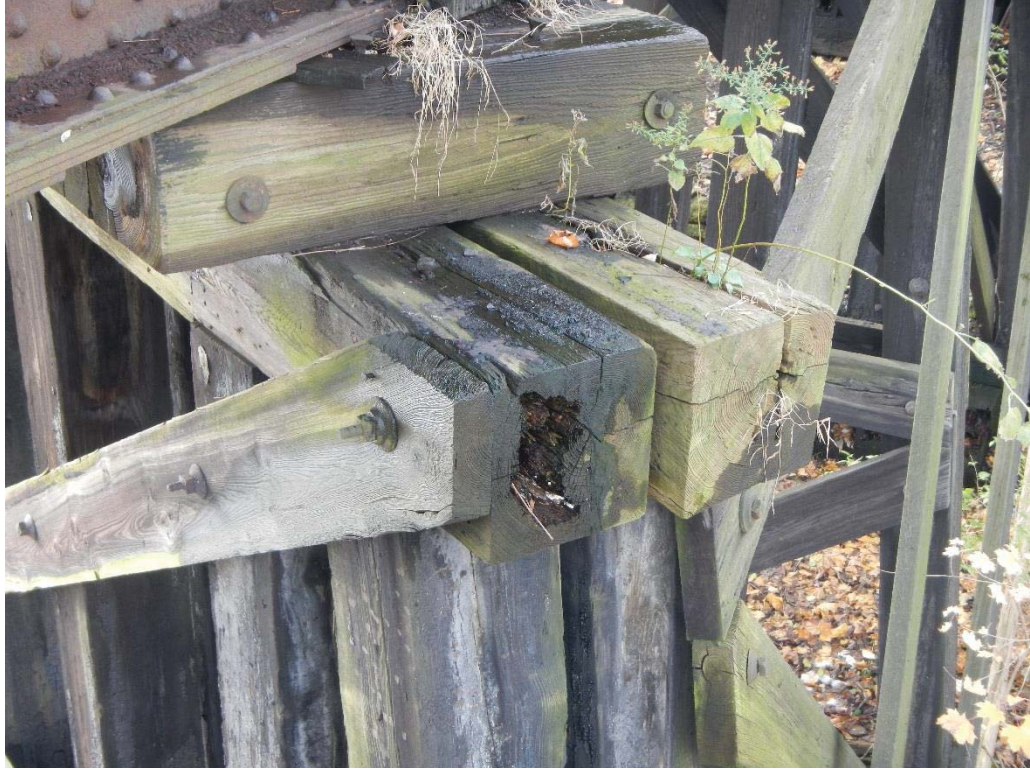
37. Pier 4 Left (North) End Top Strut Decay and Splits
