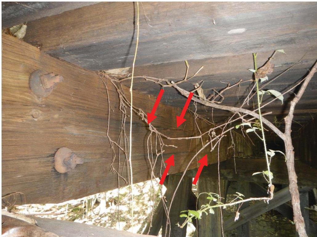
26. Span 17 Stringer 3 Horizontal Splits in Stringer
