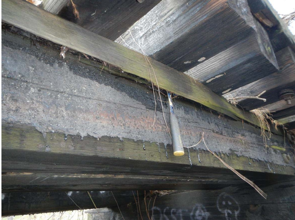
21. Span 9 Stringer 6 Decay to Top Portion of Stringer Along Entire Span
