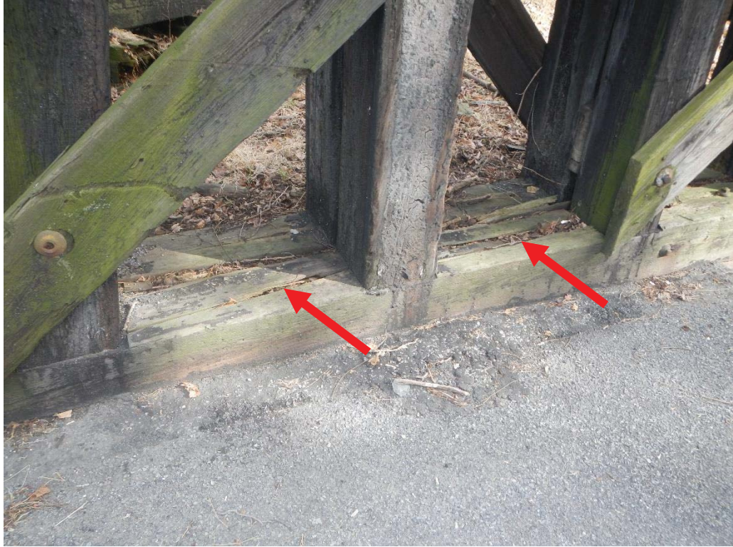
45. Pier 5 Bottom Strut Split/Decay Between Columns (Typical Condition)
