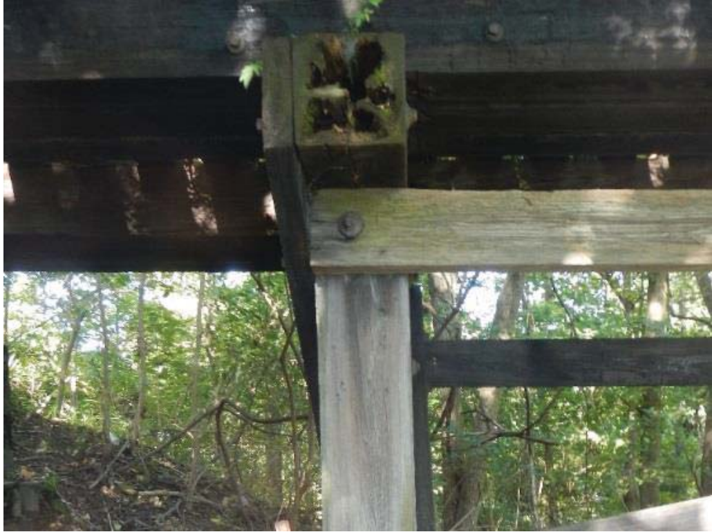
33. Pier 1 Right (South) End Top Strut Decay
