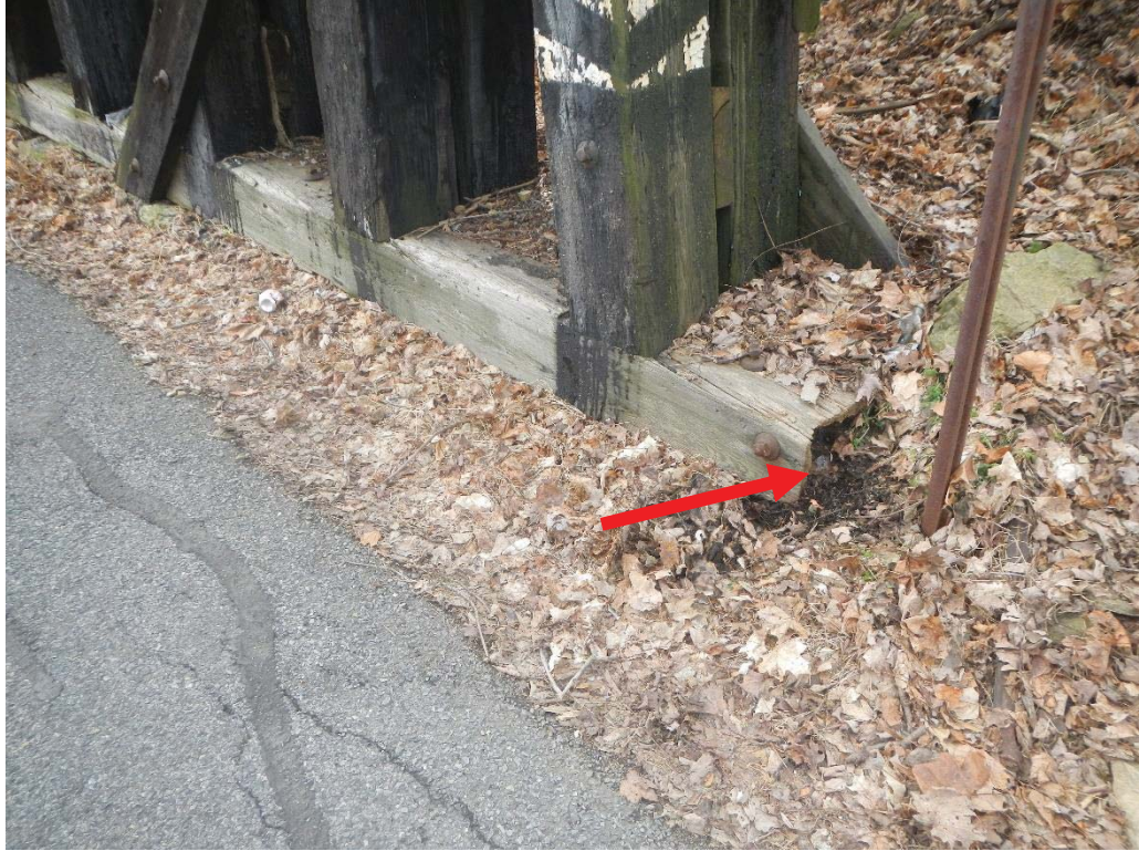
43. Pier 4 Left (North) End Bottom Strut Decay
