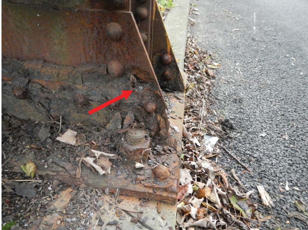
71. Pier 7 Column 1 Connection Angle 100% Section Loss
