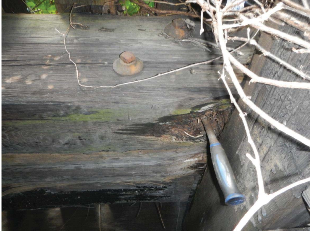
21. Span 14 Stringer 6 Decay to Bottom of Stringer Adj to Pier 14 (Hammer Penetration up to 6") (Decay Extends Full Height)
