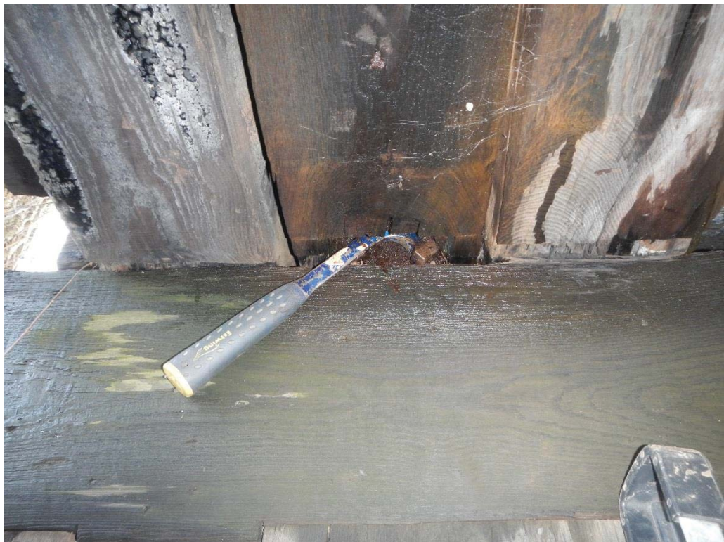
16. Span 3 Stringer 5 Decay at Bottom of Stringer Adj to Pier 2 (Hammer Penetration up to 4") (Decay Extends Full Height)
