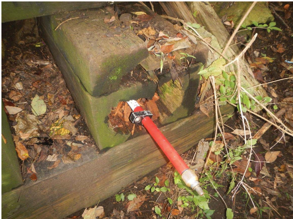
48. Pier 1 Mudsill 1 Decay Close Up (3' of Penetration with 4' Rod, Typical Condition)
