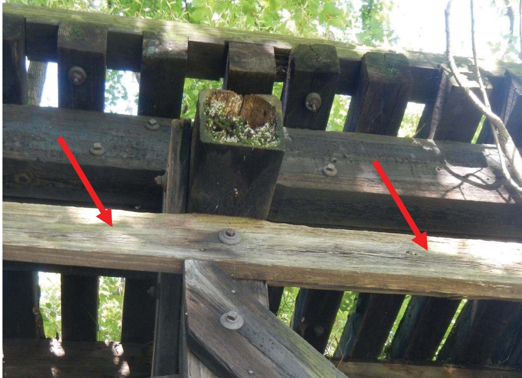
51. Spans 2 & 3 Top Right (South) Longitudinal Bracing Weathering/Decay
