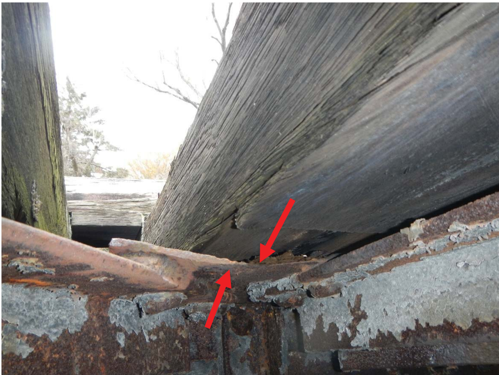
34. Span 9 Girder 1 Top Flange Horizontal Gusset Plate Bent with Section Loss between Diaphragm 2 and 3
