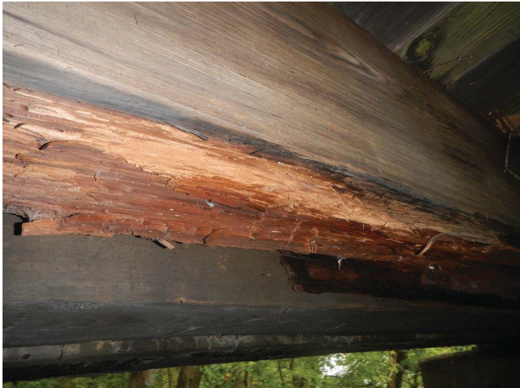
14. Span 2 Stringer 3 Decay Along Bottom of Stringer
