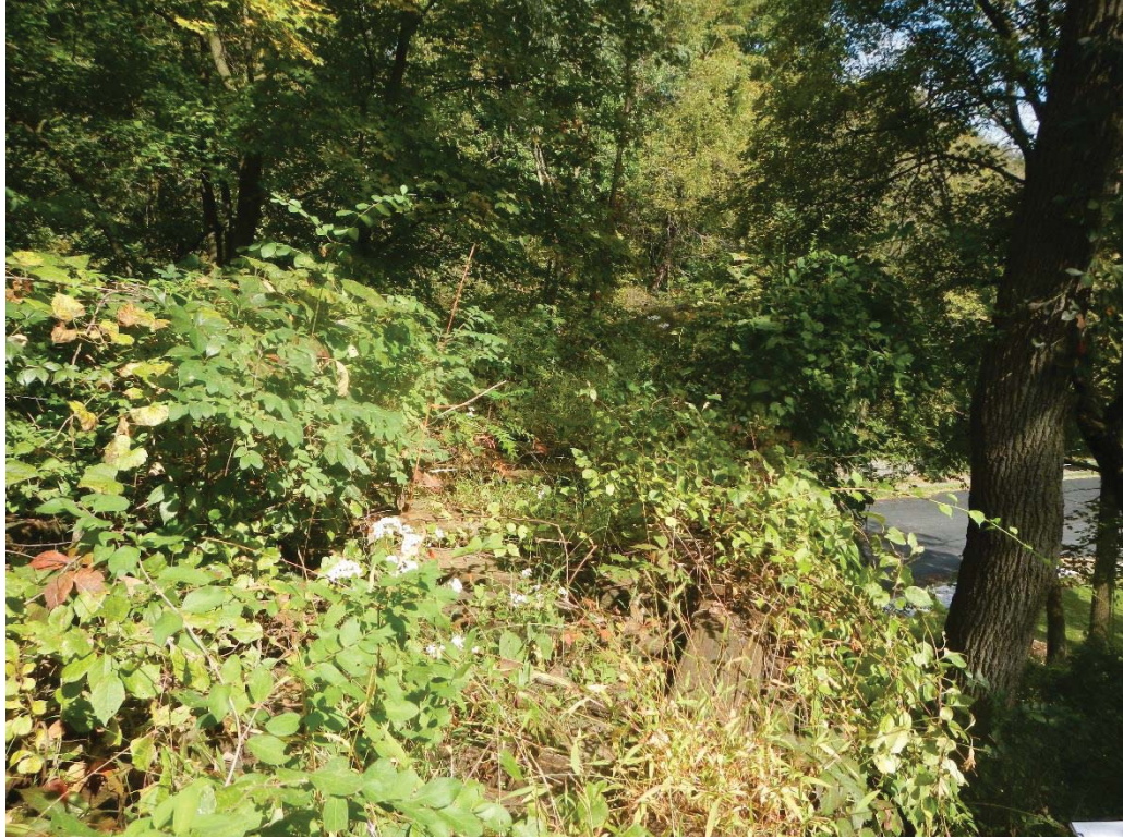
13. Significant Vegetation Growth Along Ties at Near (West) End
