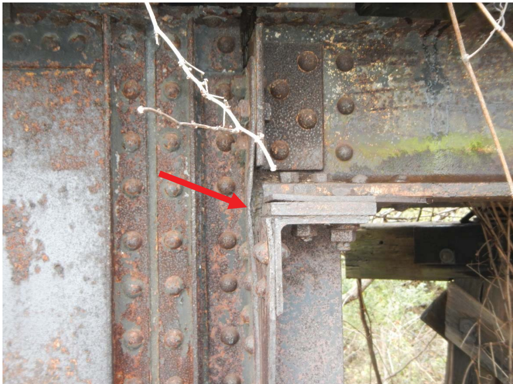
36. Span 10 Stringer 2 Bent Connection Angle with Section Loss Adjacent to Pier 9
