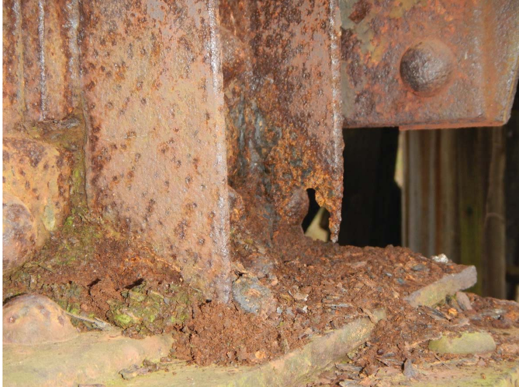
29. Span 8 Girder 1 100% Section Loss to Stiffener Adjacent to Pier 7
