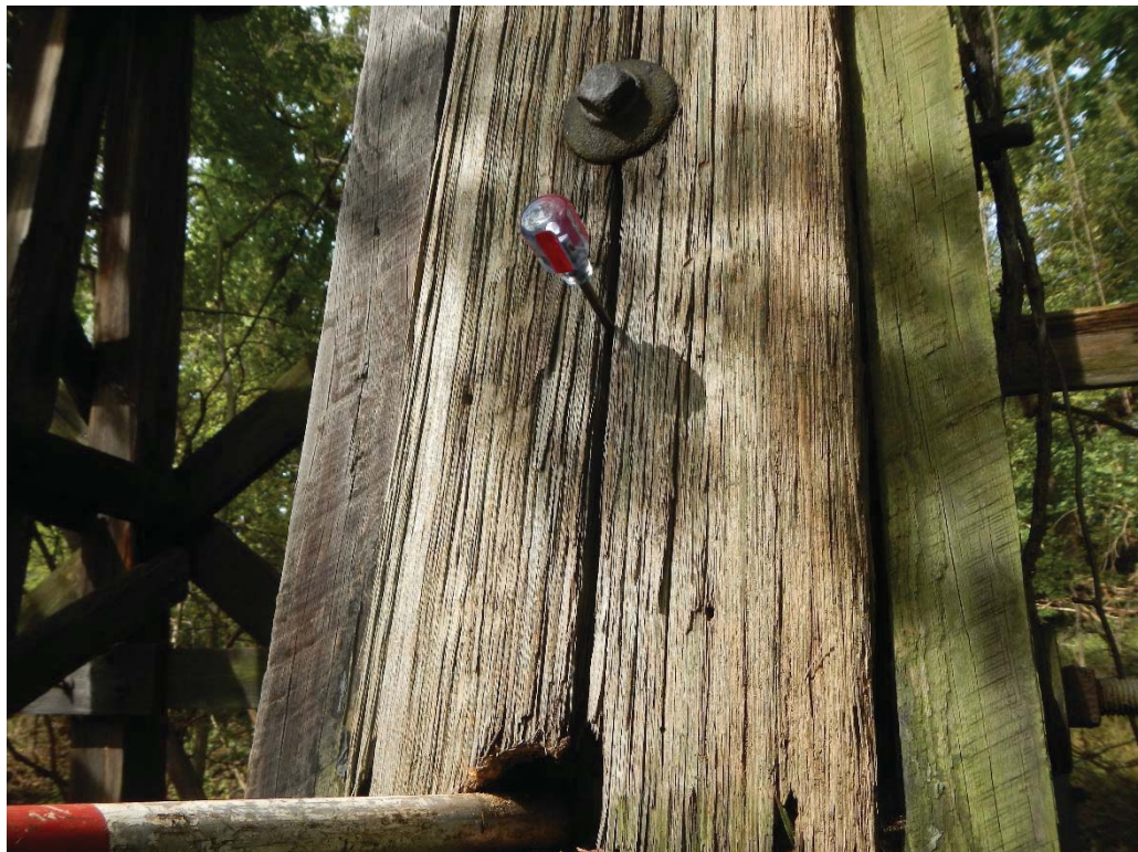
56. Pier 15 Column 4 Decay Around Column Splice Close Up
