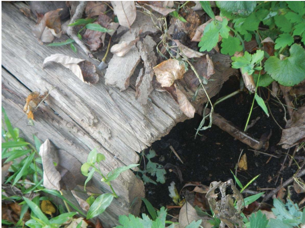
44. Pier 4 Left (North) End Bottom Strut Decay Close Up (5' of Penetration with 6' Rod)
