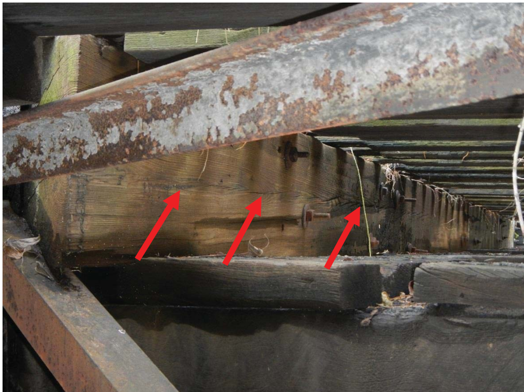
18. Span 4 Stringer 4 Horizontal Split in Stringer Adjacent to Pier 4 (Split is Full Length)
