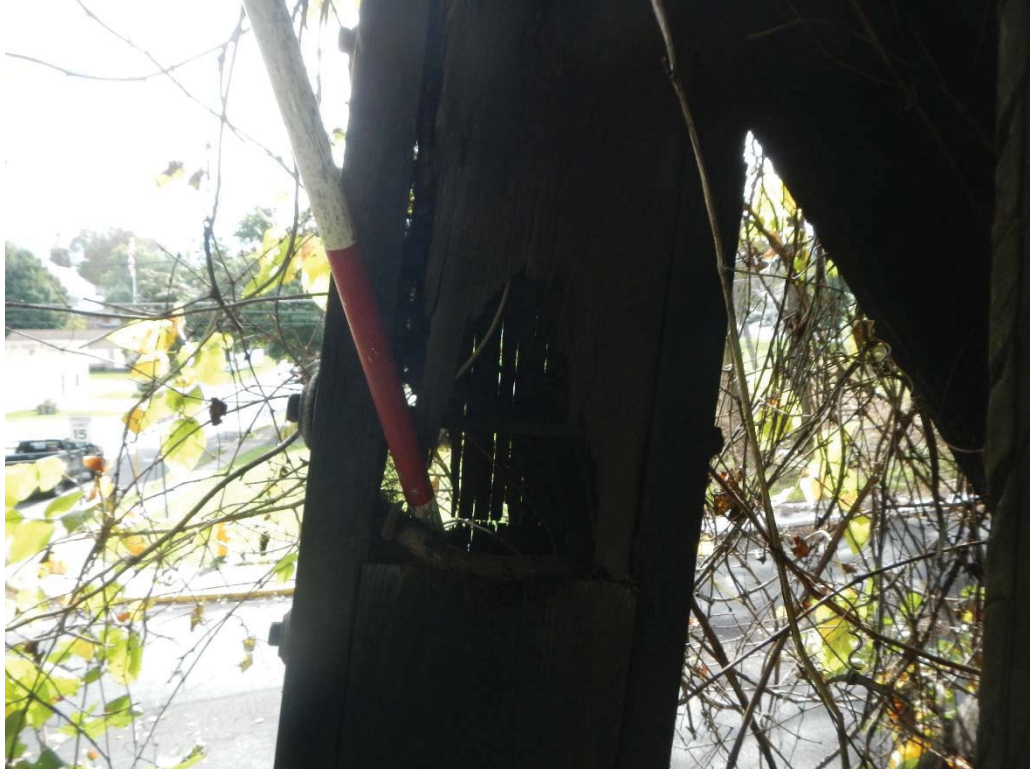
51. Pier 10 Column 5 Decay Around Column Splice
