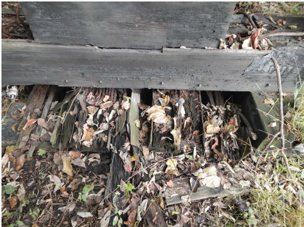
62. Pier 15 Mudsills 5 and 6 Decay Close Up
