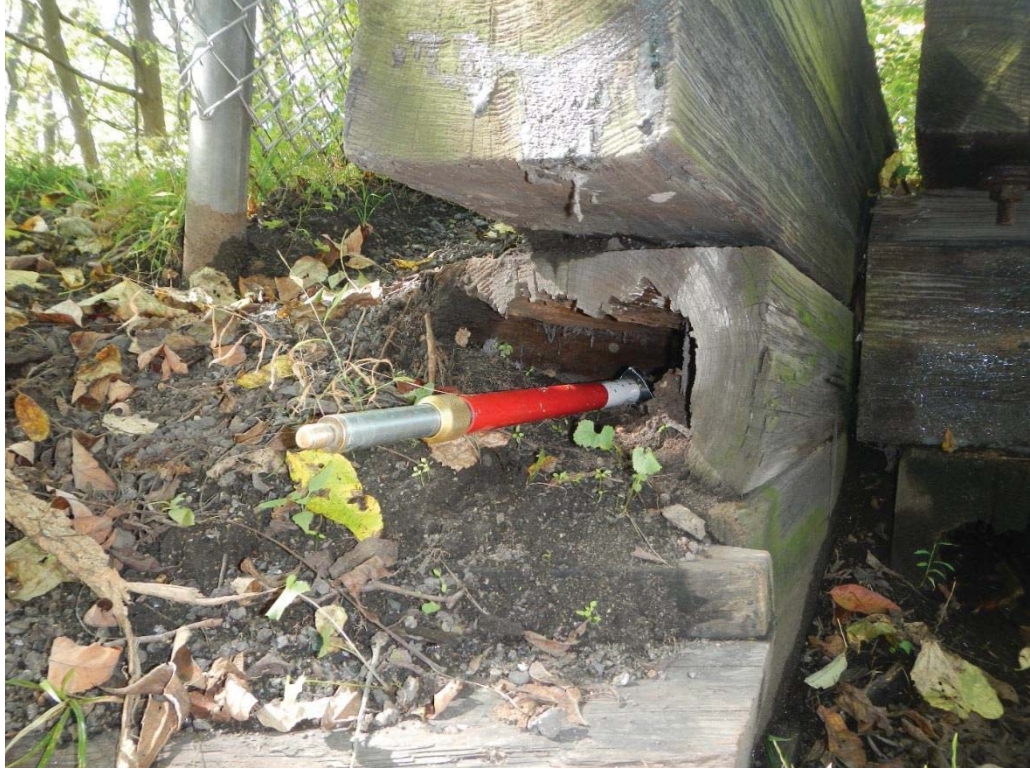
29. Near (West) Abutment Right (South) End Backwall Member Decay (4' of Penetration with 4' Rod)
