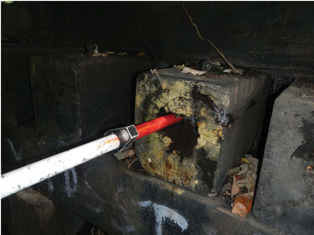
38. Far (East) Abutment Stem Longitudinal Member Decay (2'-6" of Penetration with 4' Rod)
