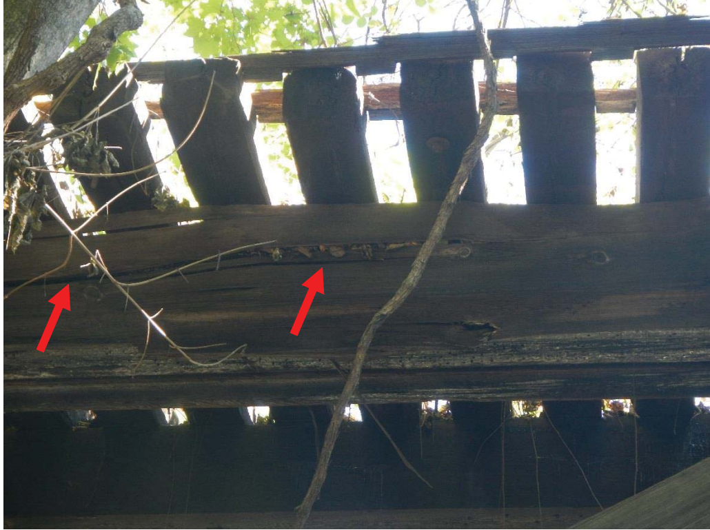
25. Span 16 Stringer 1 Decay to Top Portion of Stringer
