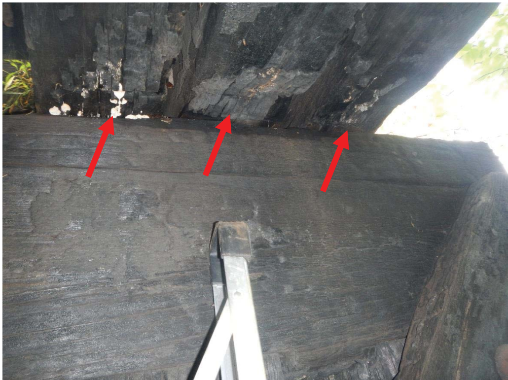
16. Span 3 Stringers 4 Thru 6 Fire/Fungus Damage Along Bottom of Stringers Adjacent to Pier 3
